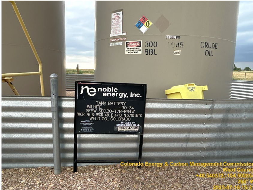
Photo #5 Wilhite 30-34, Wagner 30-32 Battery site Inactive | Shut-down Battery signage 1
