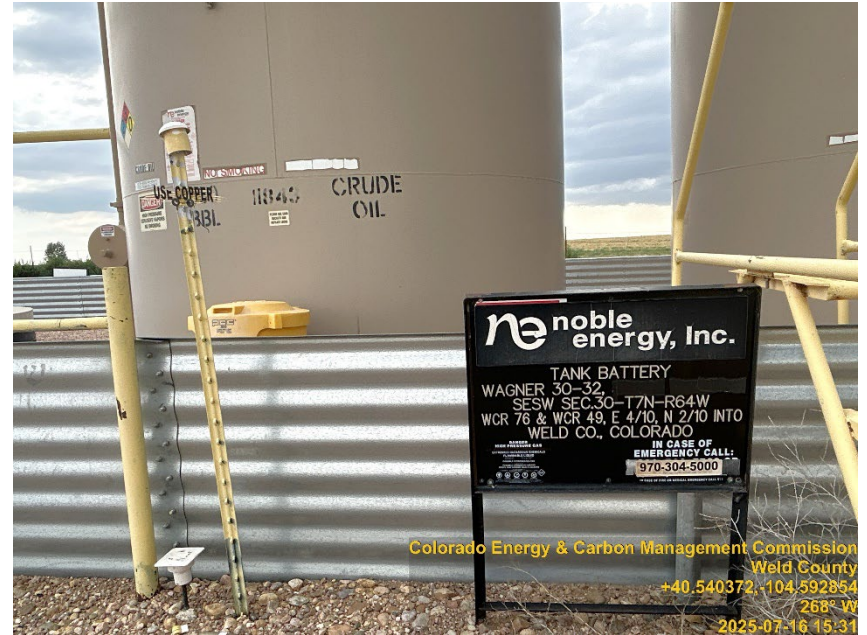
Photo #6 Wilhite 30-34, Wagner 30-32 Battery site Inactive | Shut-down Battery signage 2
