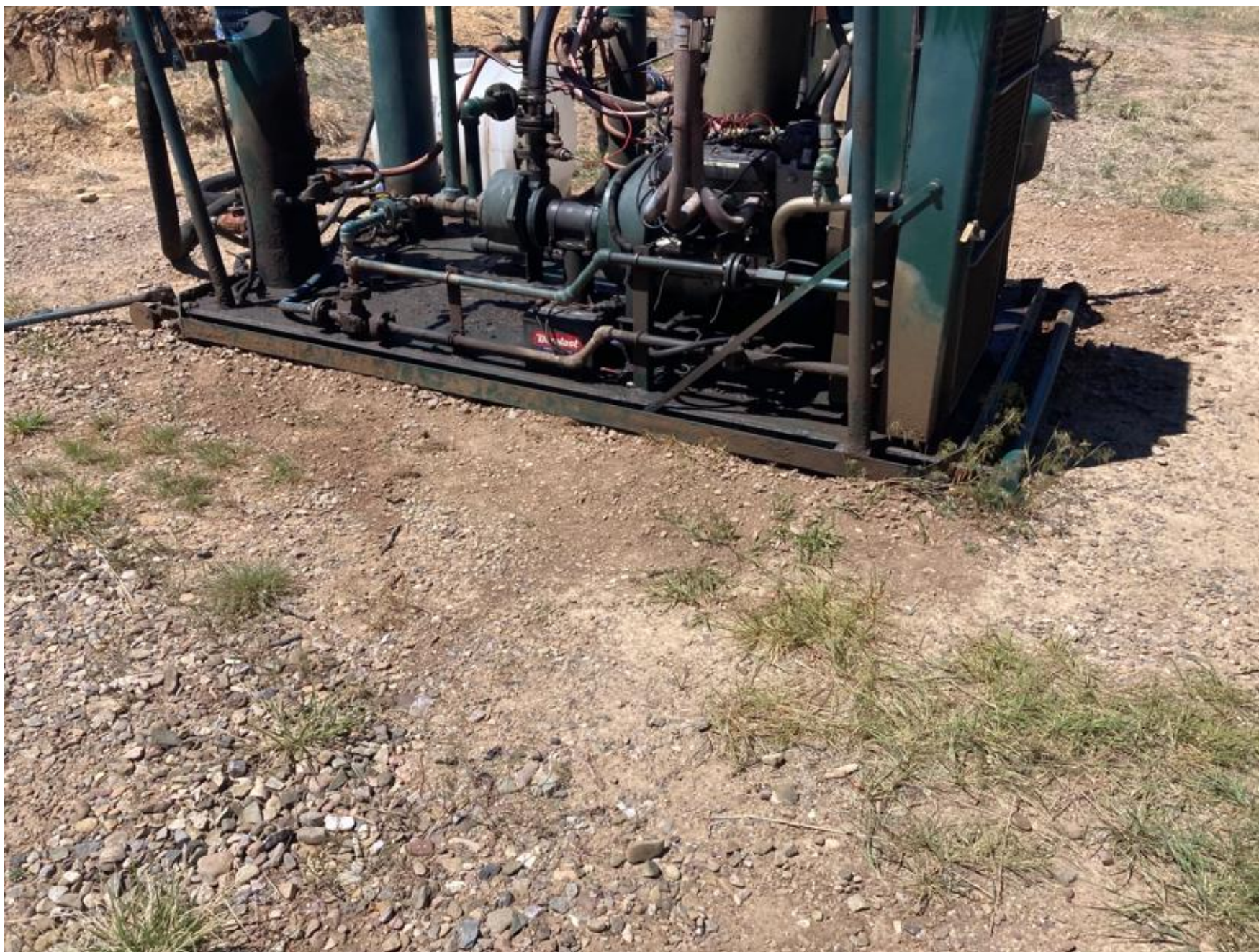
PHOTO 1: THE IMPACTED SOIL NEAR THE COMPRESSOR HAS BEEN REMOVED AND REPLACED WITH FRESH PAD MATERIAL. THE SKID HAS ALSO BEEN CLEANED. EQUIPMENT MAINTENANCE HAS BEEN PERFORMED AND THE SELF INSPECTION PROCESS REVIEWED.
