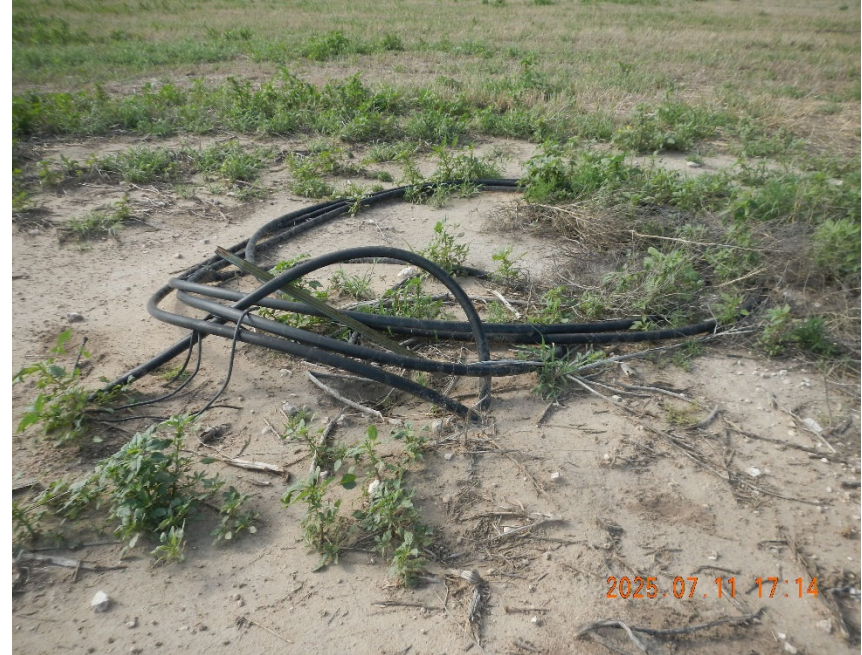
4. View of black poly line that appears to be three phase power at wellhead.
