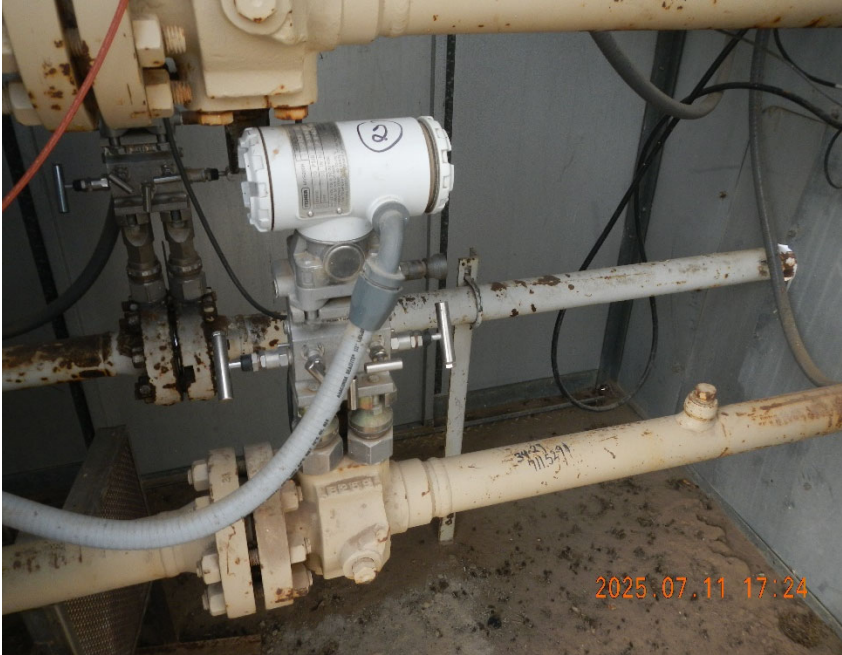
7. Gas meter inside shared meter shed.
