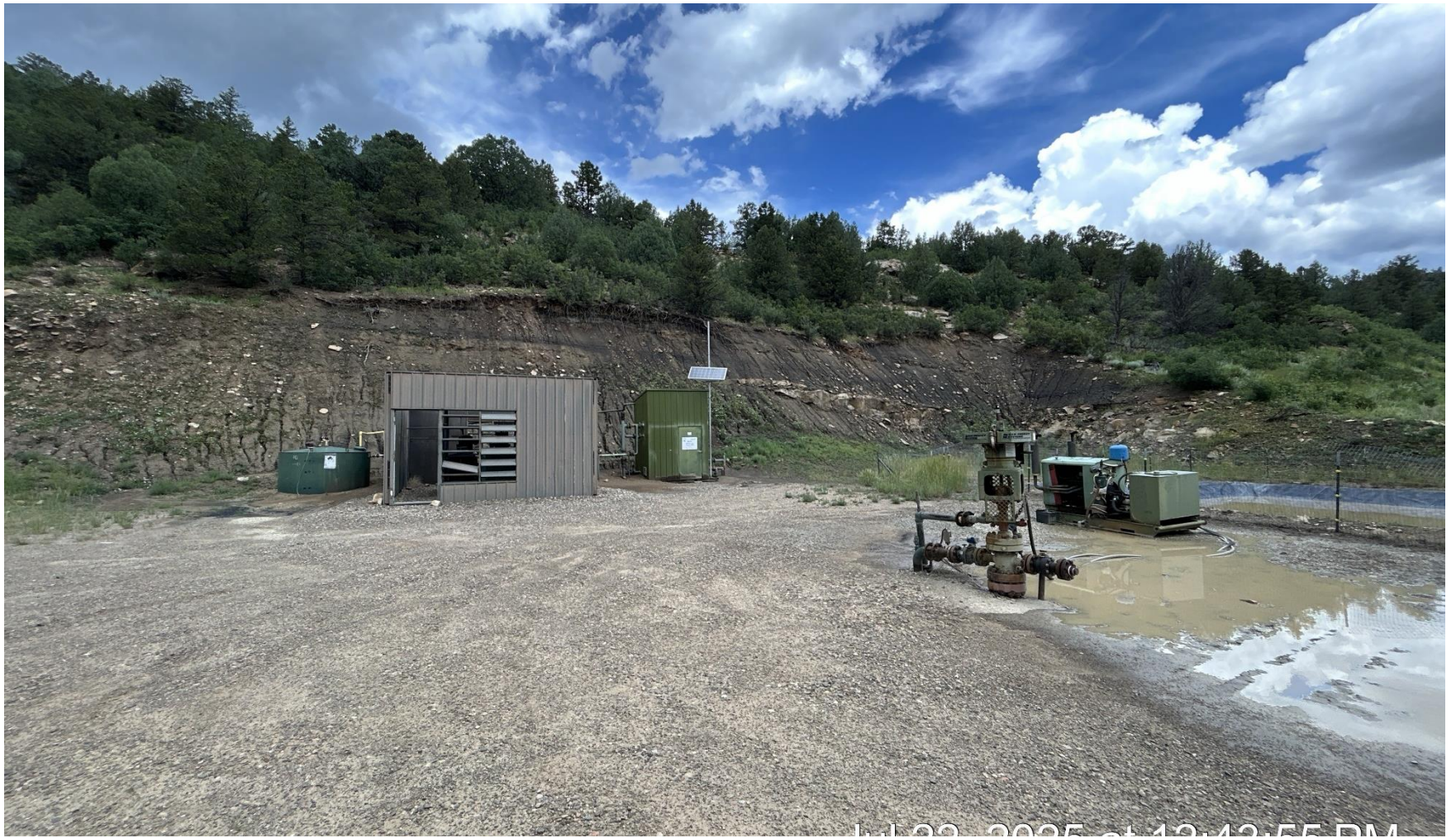
PHOTO 3: WELLHEAD AND EQUIPMENT
