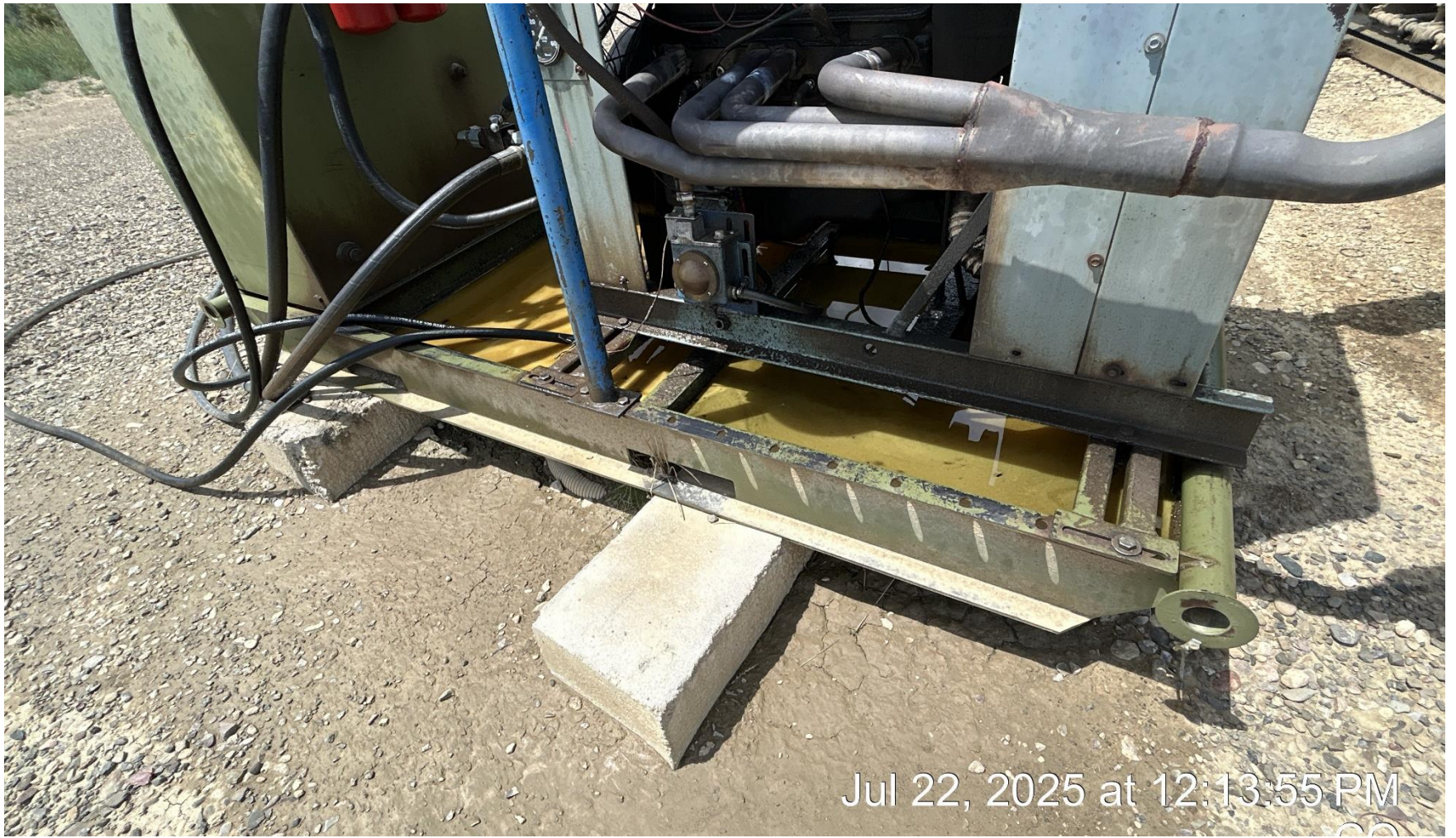
PHOTO 3: IMPACTED SOIL & SKID HAS OIL
