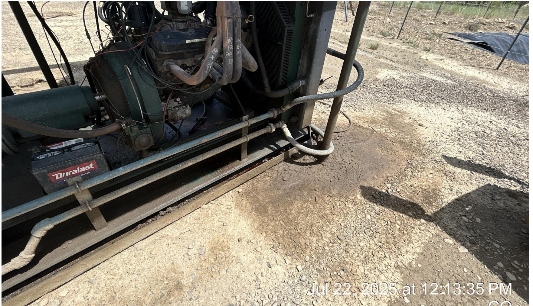
PHOTO 3: IMPACTED SOIL AT RING
