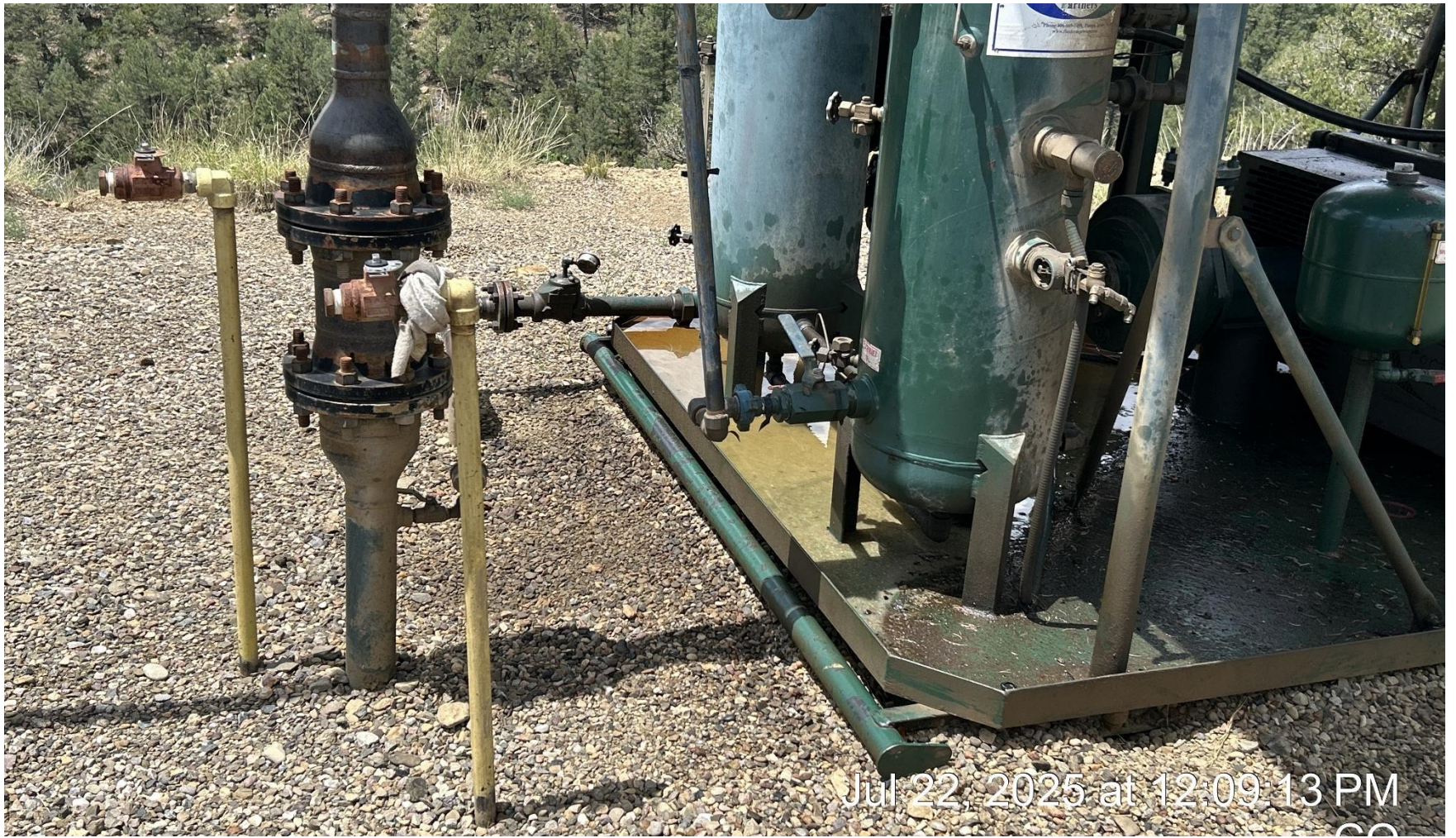
PHOTO 3: Impacted soil at ring
