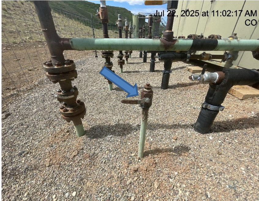
Photo # 3541 Unused flowline lacks lockout tagout (OOSLAT)
