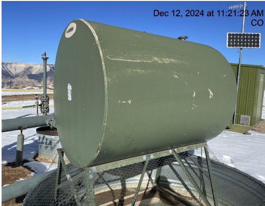
Photo # 3392 From inspection 708905234 conducted on 12/12/2024 Methanol tank improperly labeled/missing some required information
