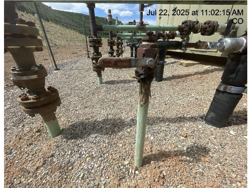
Photo # 3542 Unused flowline lacks lockout tagout (OOSLAT)
