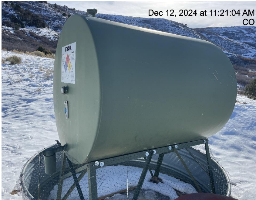
Photo # 3391 From inspection 708905234 conducted on 12/12/2024 Methanol tank improperly labeled/missing some required information
