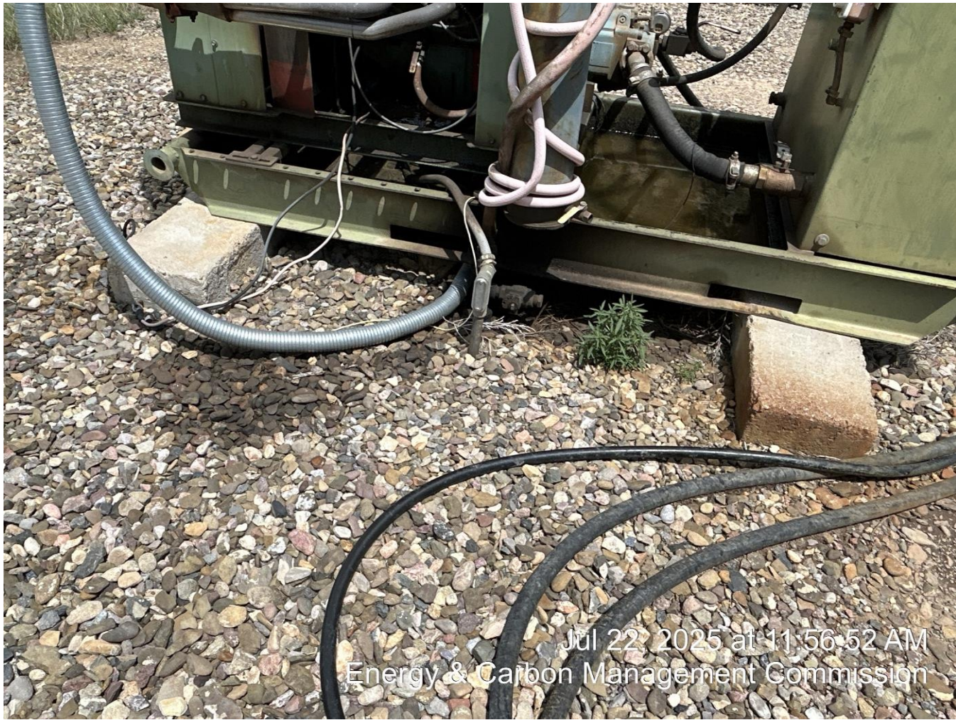
PHOTO 4: Impacted soil at Skid
