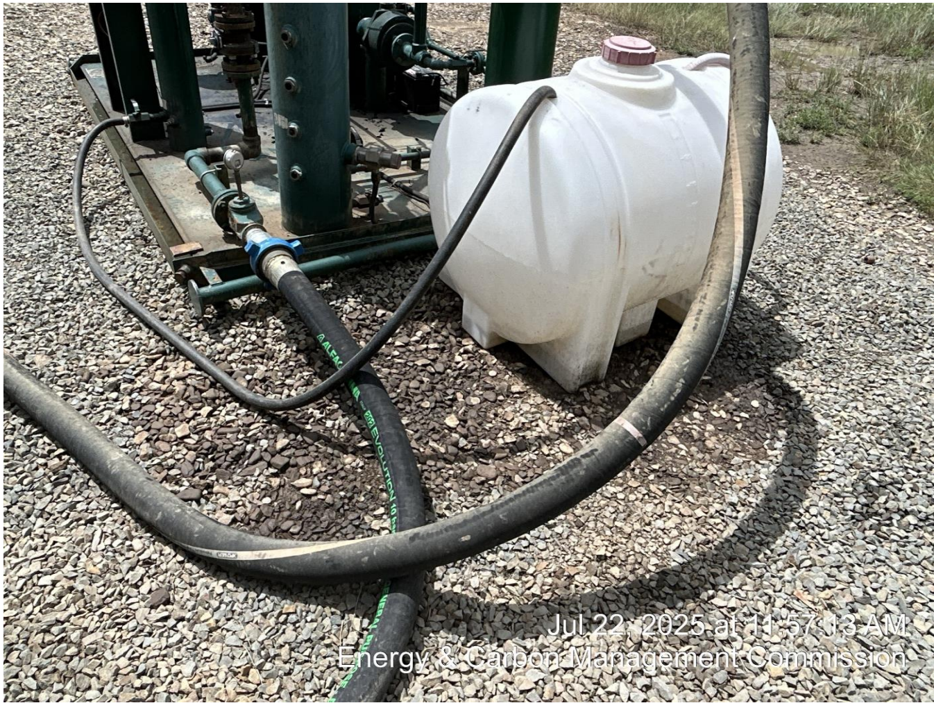
PHOTO 5: Impacted soil at ring
