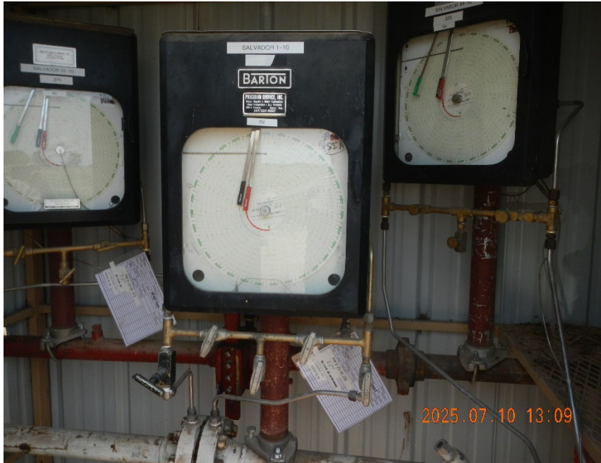
5. Gas meter inside meter shed.
