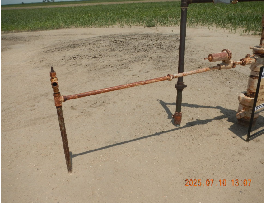
3. View of Domestic Tap at wellhead.
