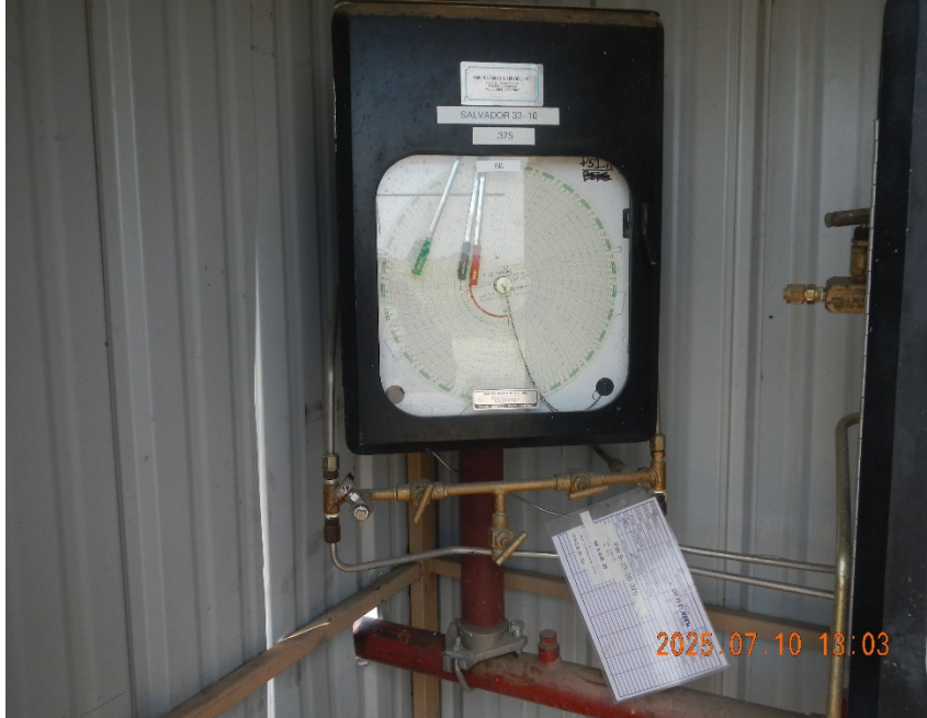
5. Gas meter inside meter shed.
