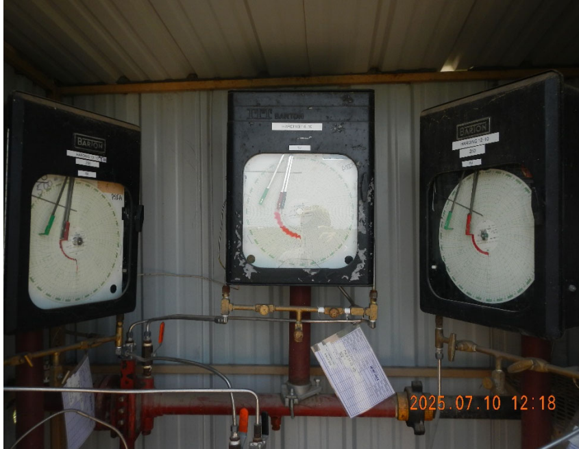
5. Gas meter inside meter shed.
