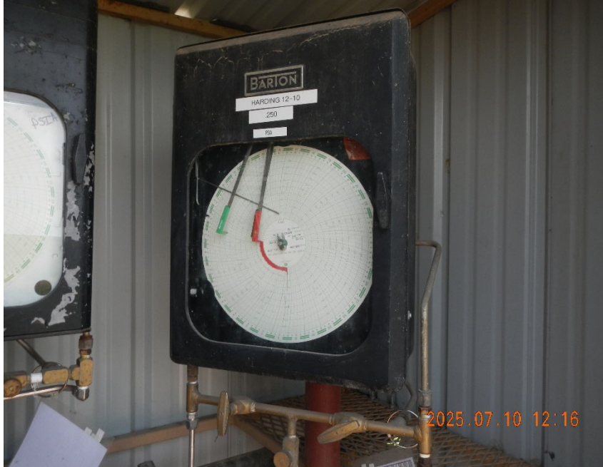
5. Gas meter inside meter shed.
