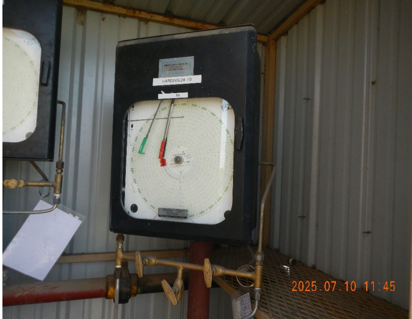
5. Gas meter inside meter shed.
