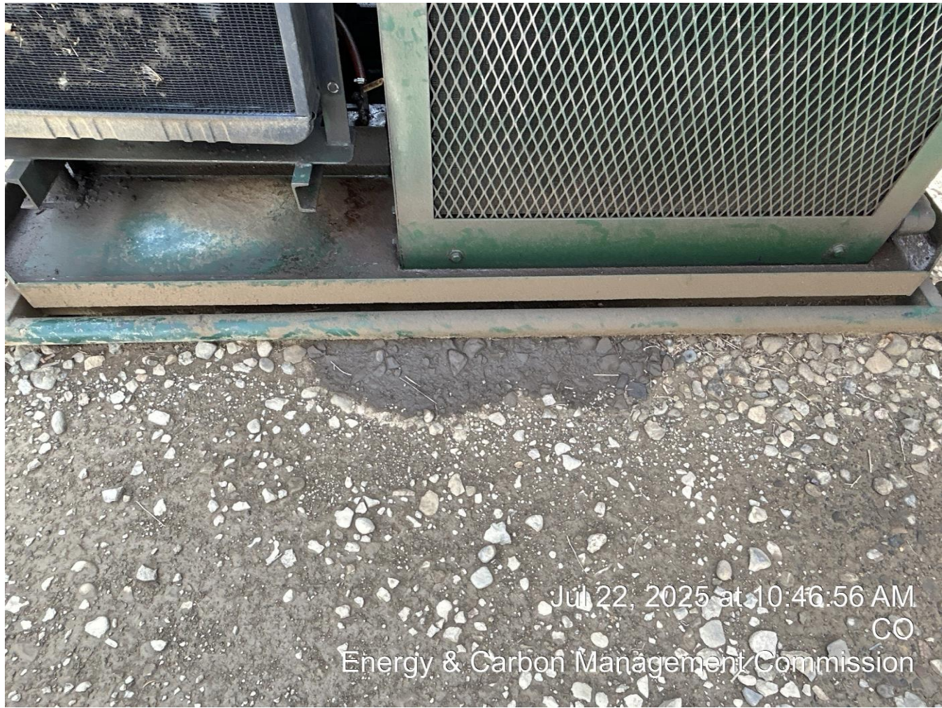
PHOTO 5: Impacted soil front of liquid ring
