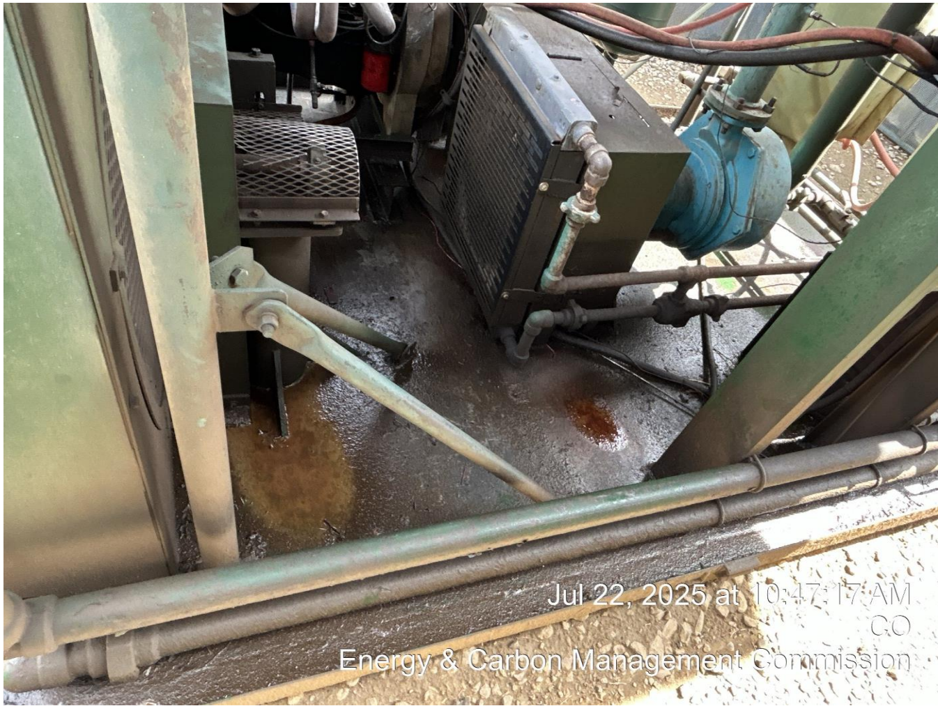
PHOTO 6: Liquid ring engine has oil leaks
