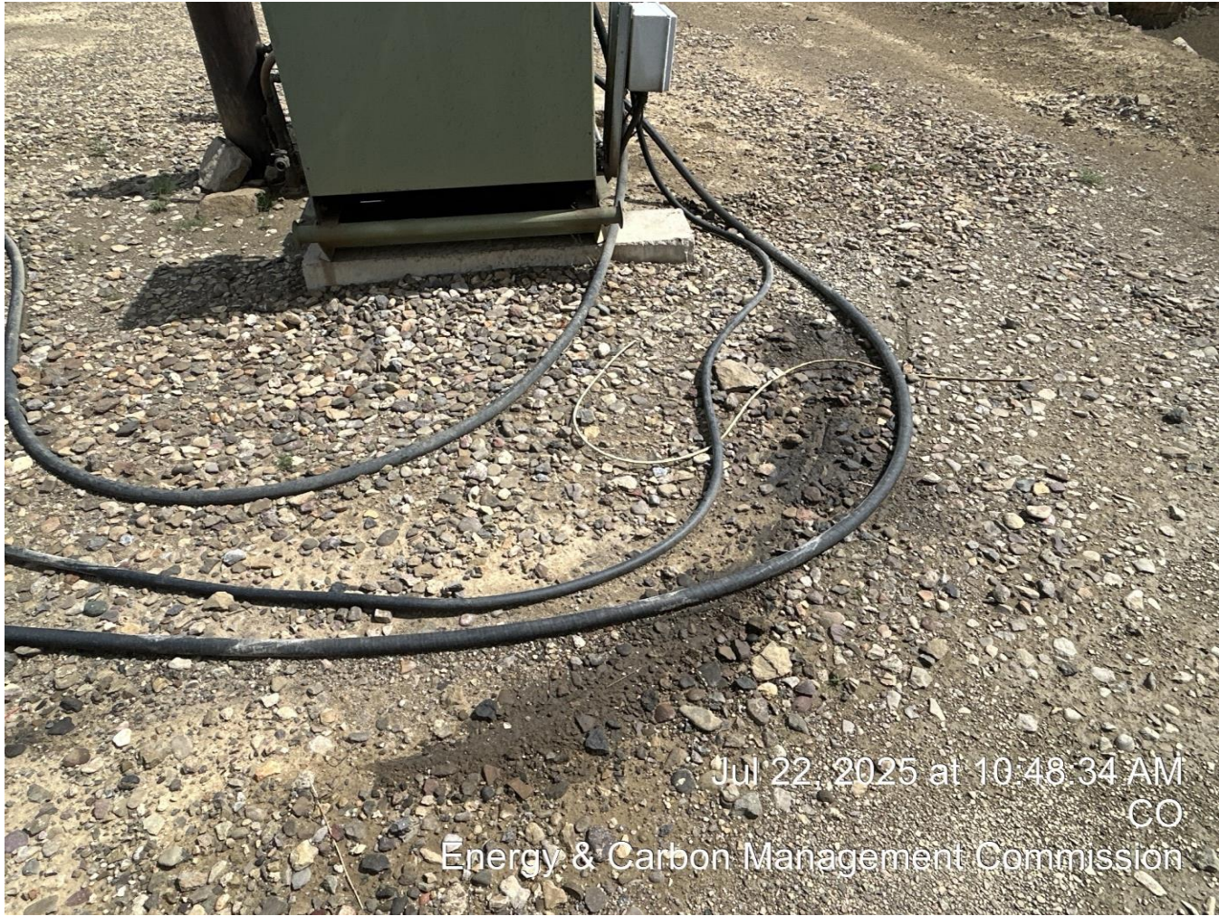
PHOTO 4: Impacted soil at drive head hoses
