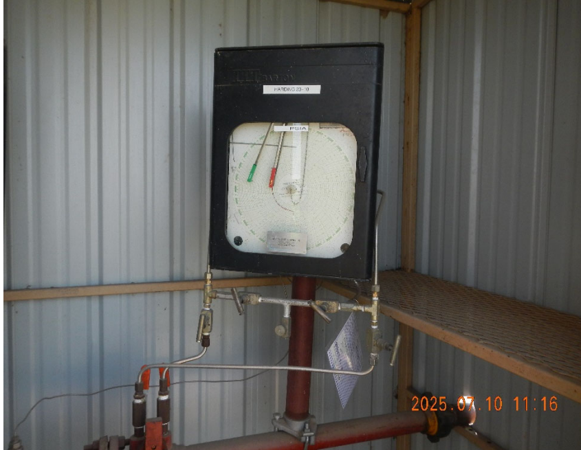
5. Gas meter inside meter shed.
