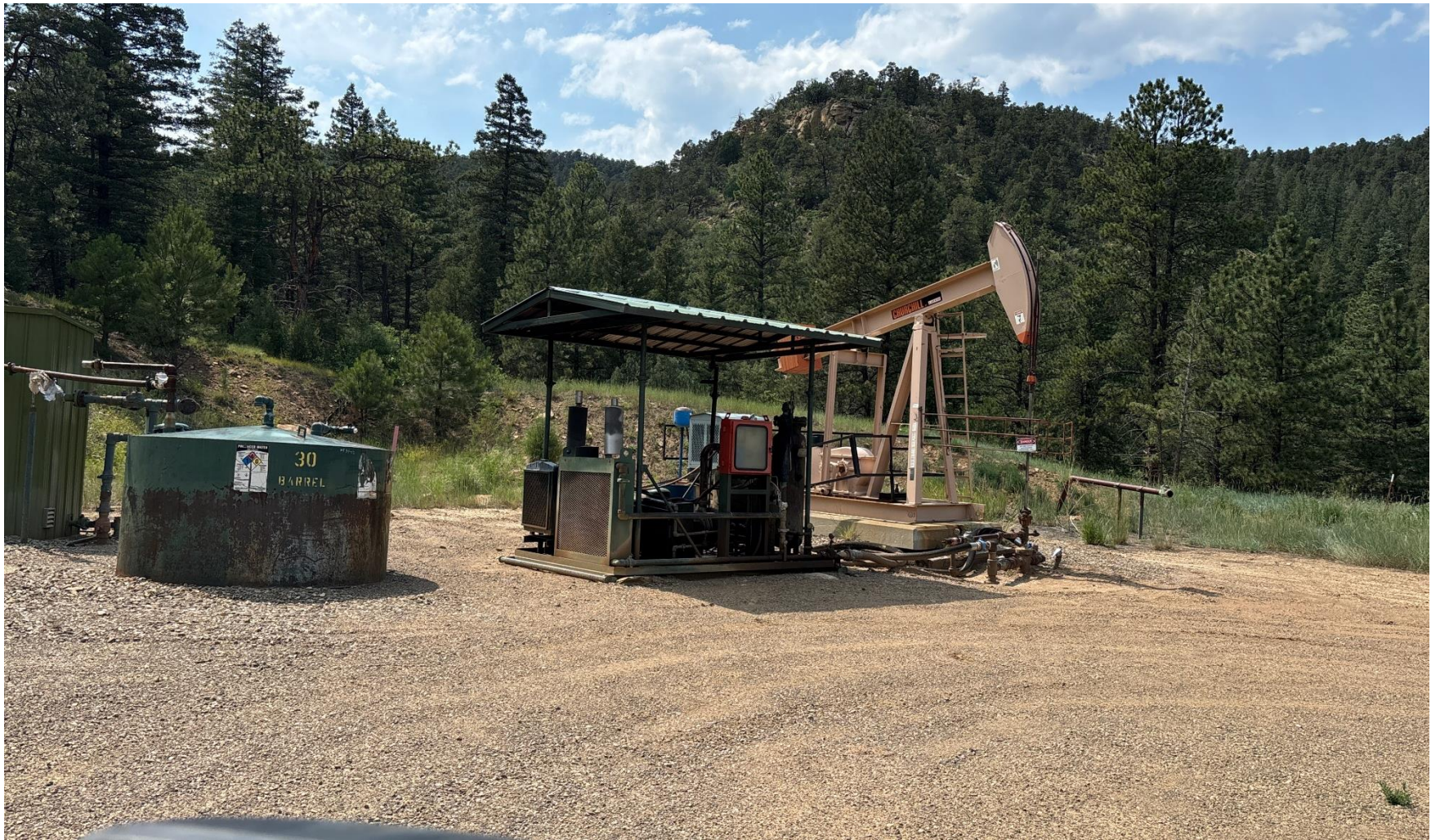
PHOTO 3: WELLHEAD AND EQUIPMENT.
