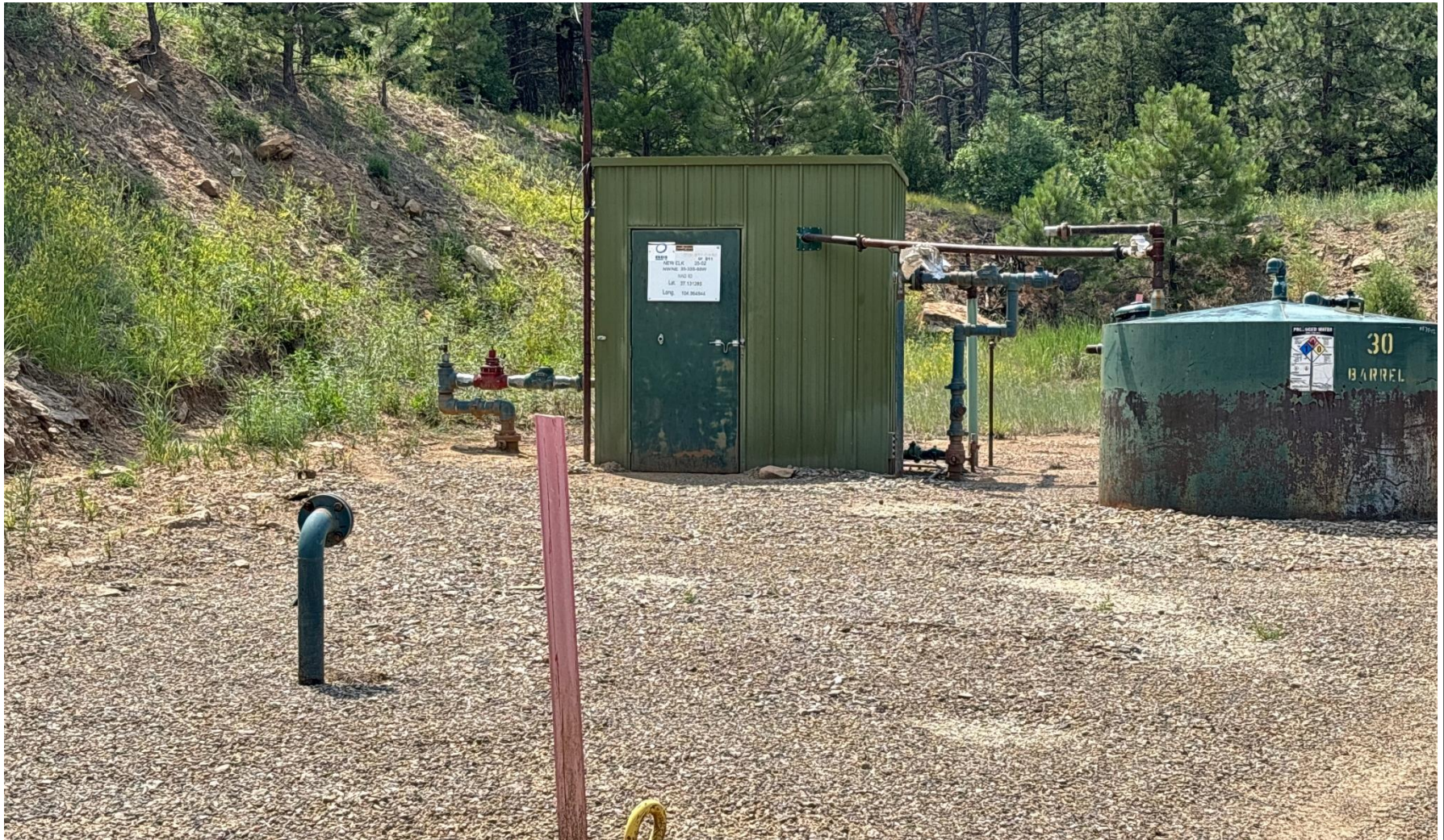
PHOTO 5: UNUSED EQUIPMENT (3" RISER NOT IN USE OR MARKED). REMOVE OR MARK 3" RISER PER RULE 606.
