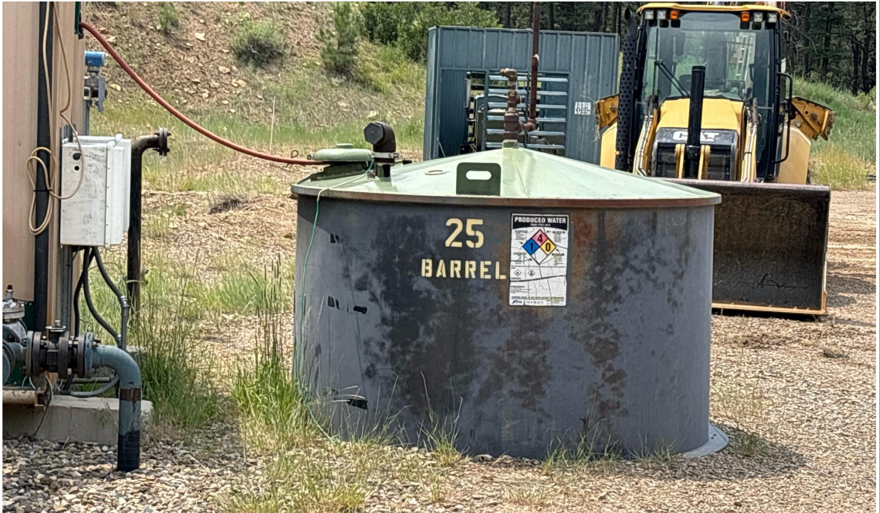
PHOTO 6: 25 BBLs PRODUCED WATER TANK.
