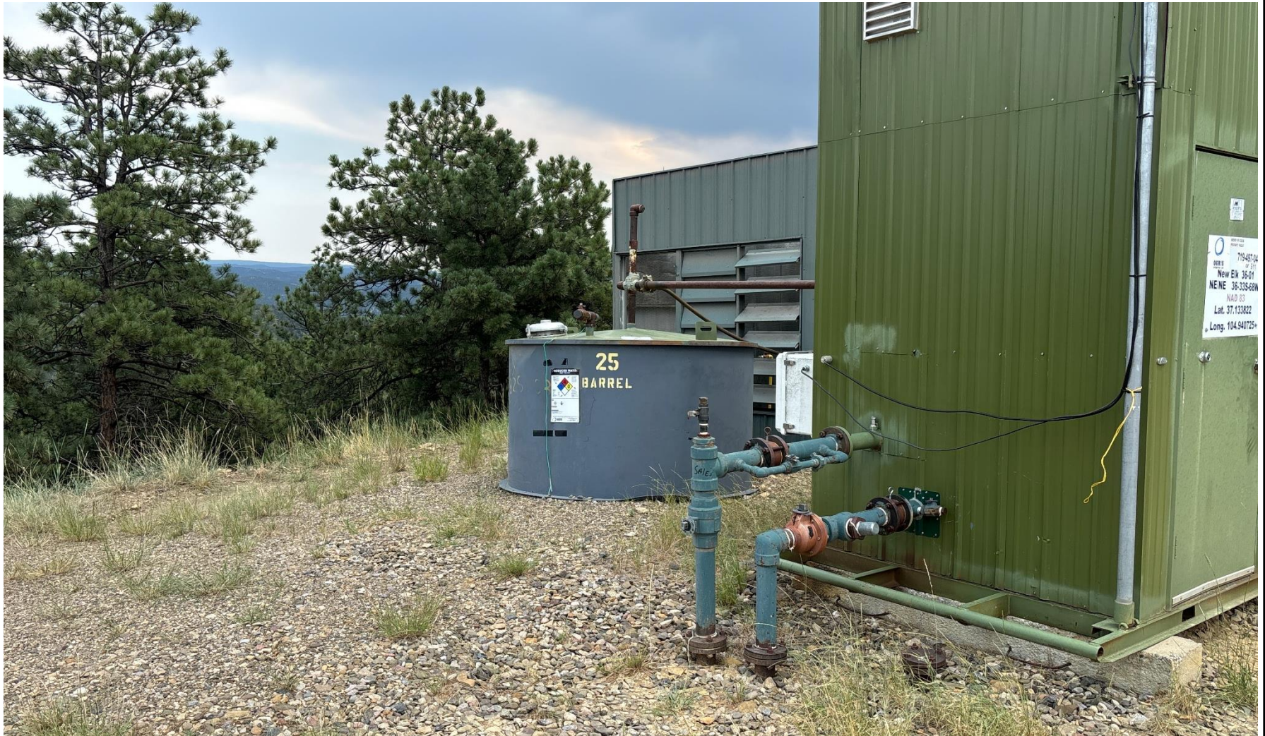
PHOTO 4: 25 BBL PRODUCED WATER TANK.
