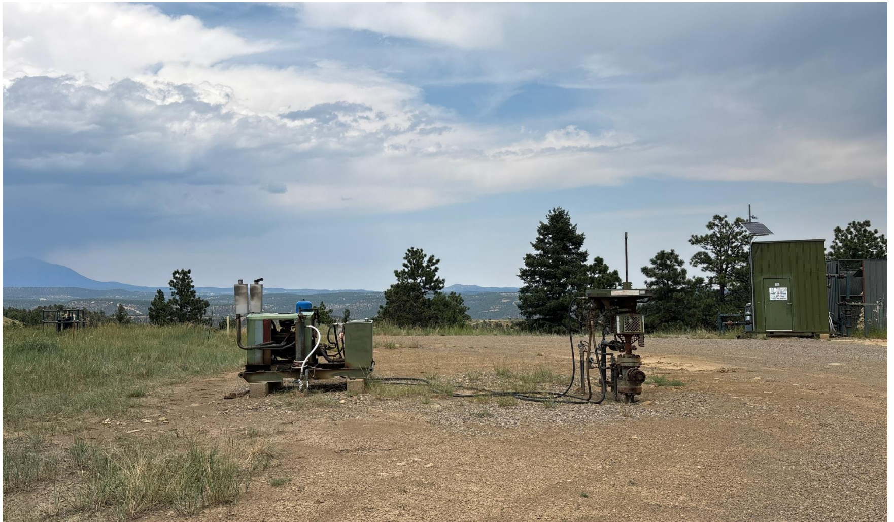
PHOTO 3: WELLHEAD AND EQUIPMENT.
