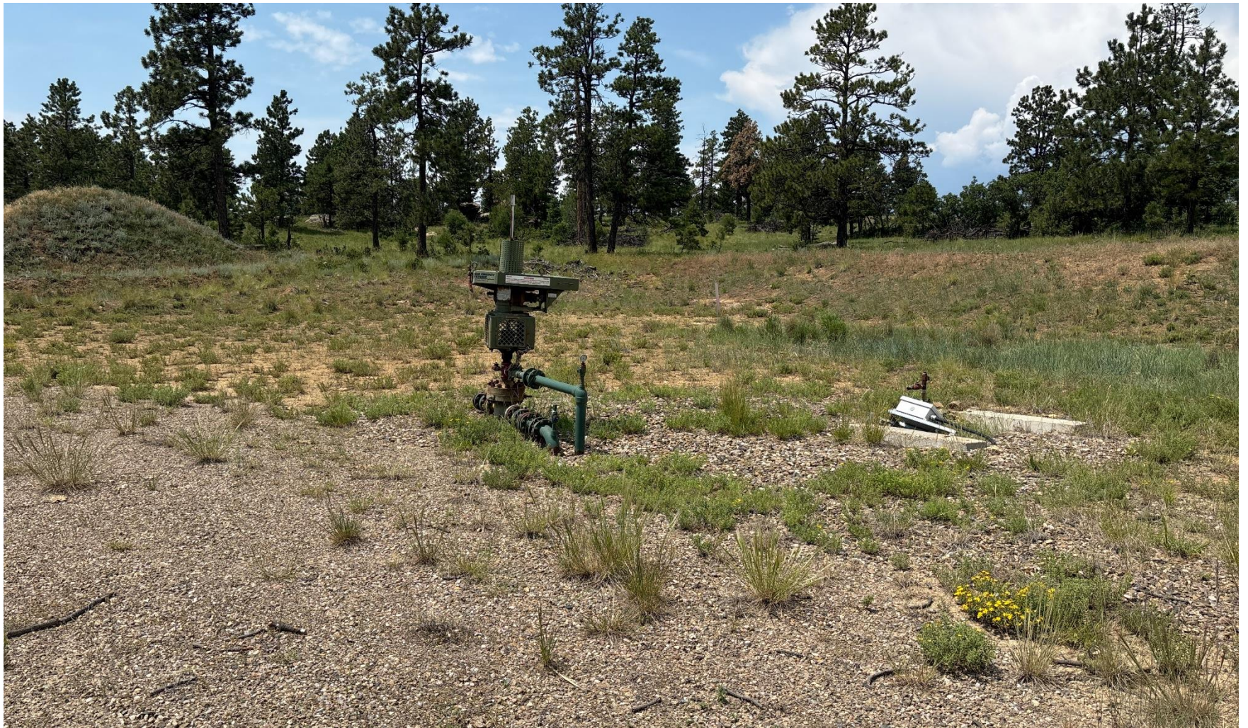
PHOTO 3: WELLHEAD AND EQUIPMENT.
