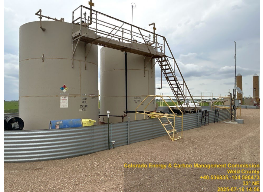
Photo #5 Faulkner 30-44 Battery site Inactive | Shut-down Equipment documented: Loc. ID 306393
