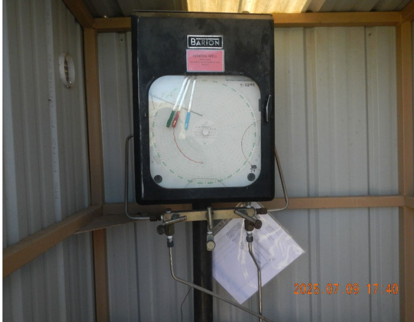
3. Gas Meter inside Meter Shed.
