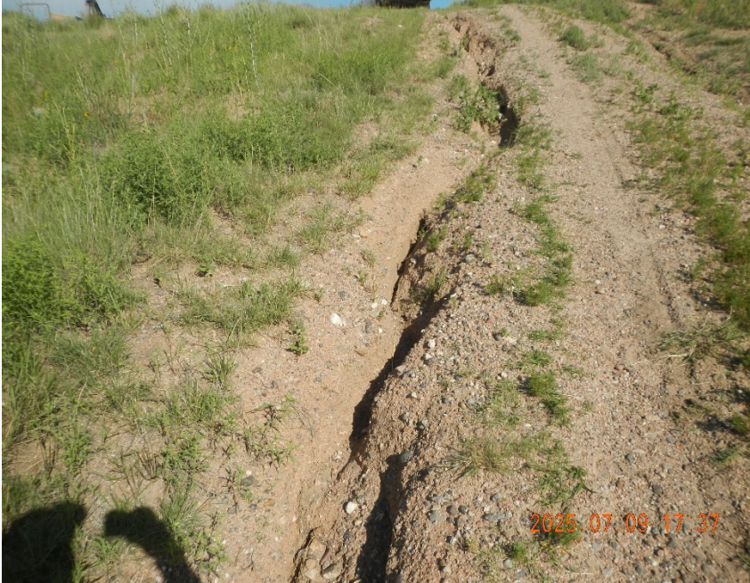
9. Closer view of erosion along access trail.
