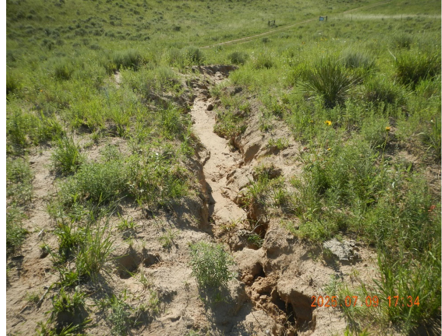
10. Erosion at edge of location looking down grade.
