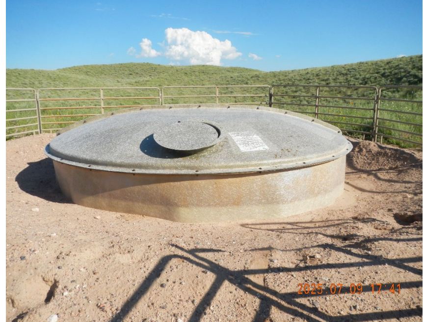
4. View of produced water tank.
