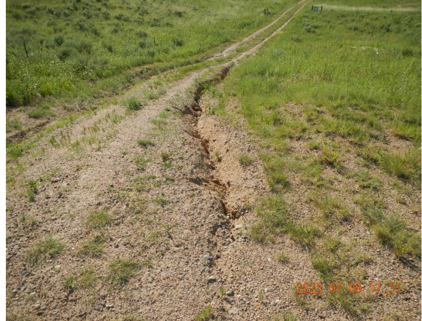
8. Erosion on access trail looking down from well location.
