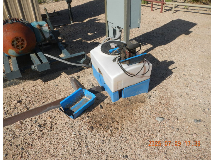
6. Disconnected tank and pump at well location with stained soil around bottom of tank.
