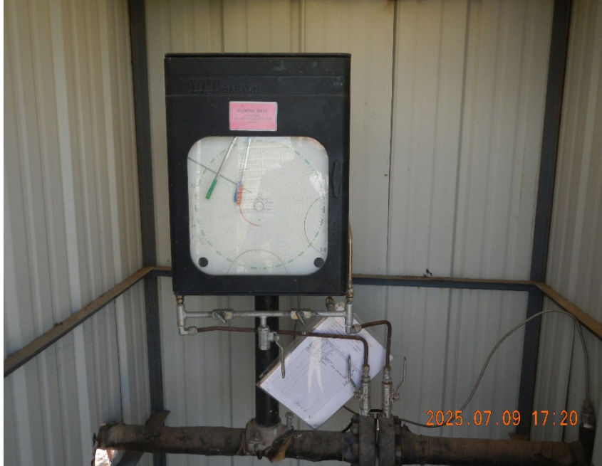
3. Gas Meter inside Meter Shed.
