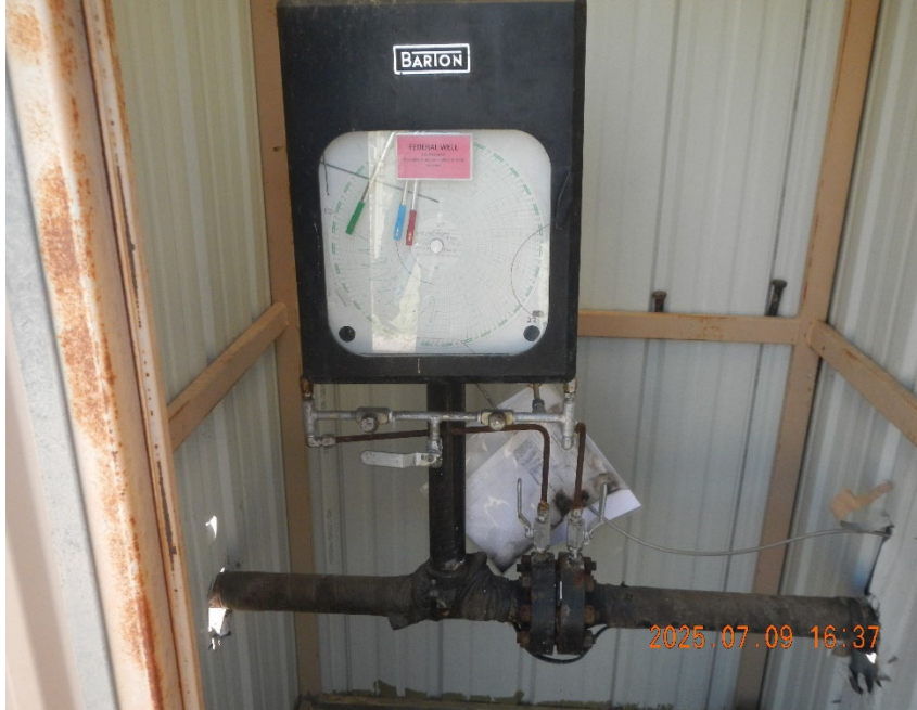
3. Gas Meter inside Meter Shed.
