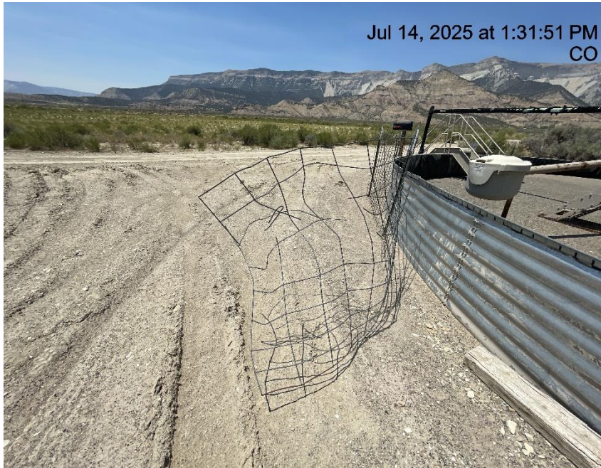
Photo # 2129 Hog panels around tank battery damaged
