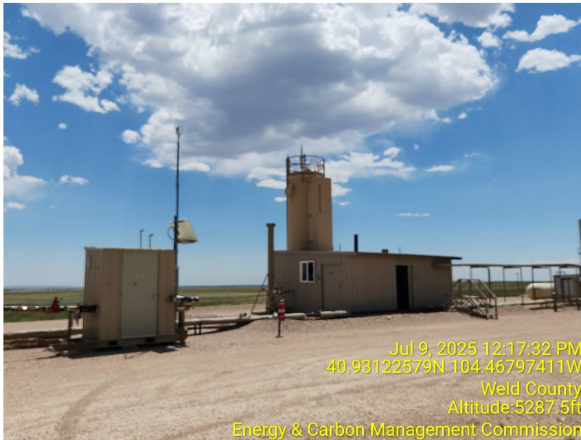
Photo 5 – Gas Meter and Heater Treater
