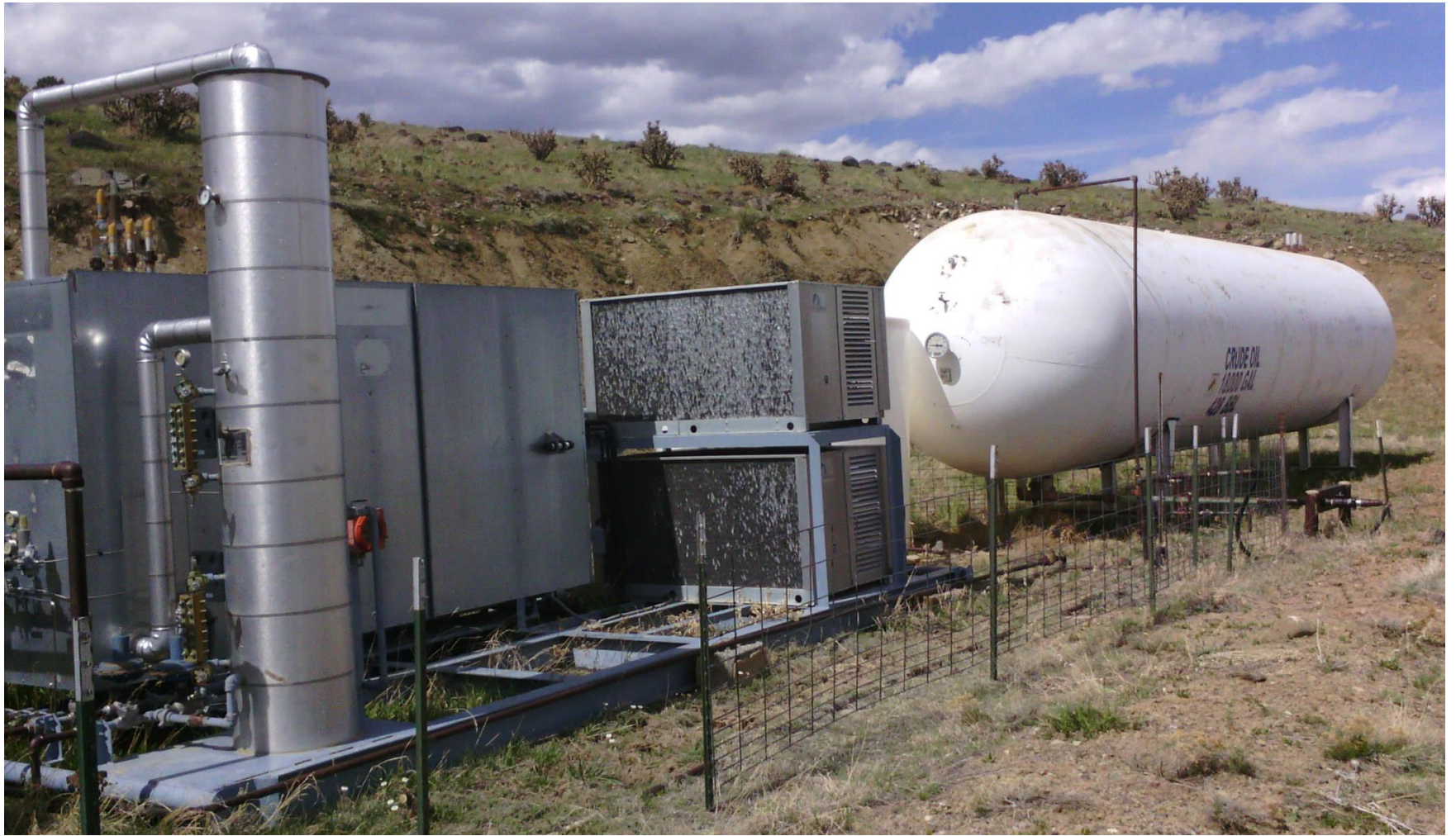
PHOTO @: Unused Equipment
