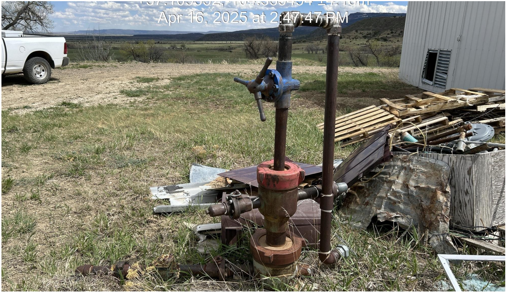
PHOTO 3: WELLHEAD No Sign
