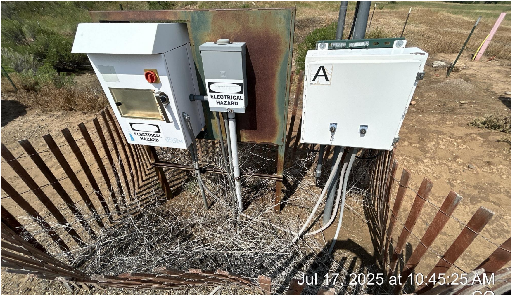
PHOTO 3: WEEDS IN ELECTRICAL EQUIPMENT
