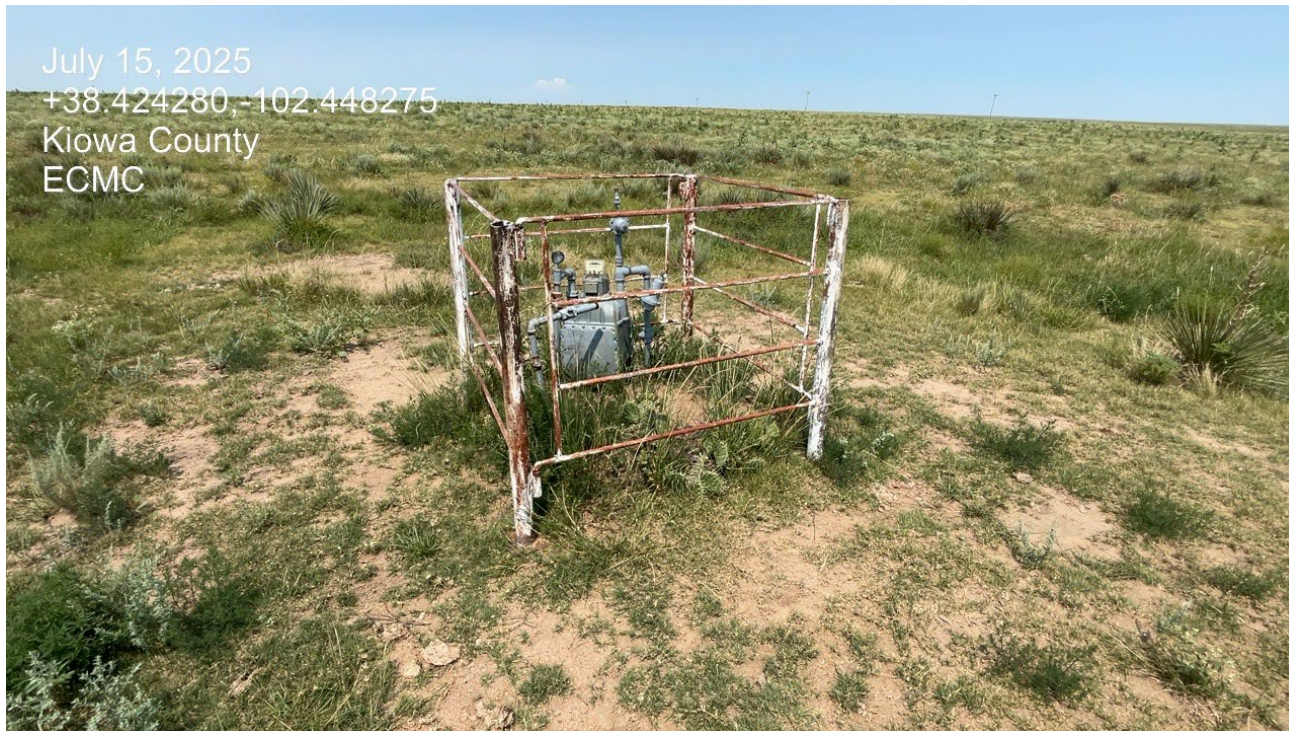
Photo 4. There is a pipe riser/gas meter on location that was never removed.
