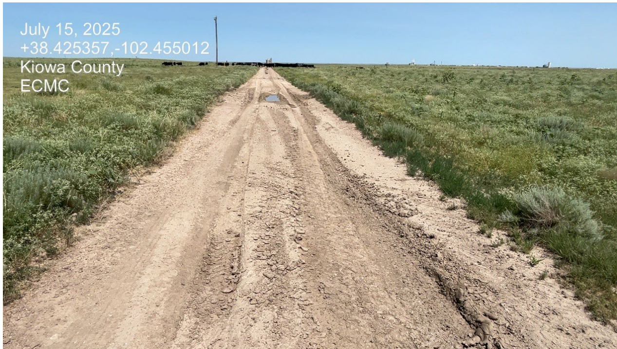
Photo 1. Facing north along the access road. There are areas of vehicle rutting that need to be repaired and stabilized with gravel.
