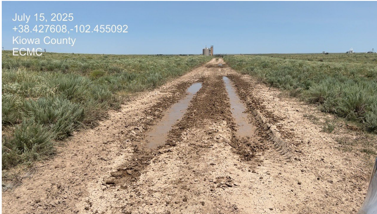
Photo 3. Facing north further along the access road. Areas accumulating stormwater need to be built up with roadbase and gravel.
