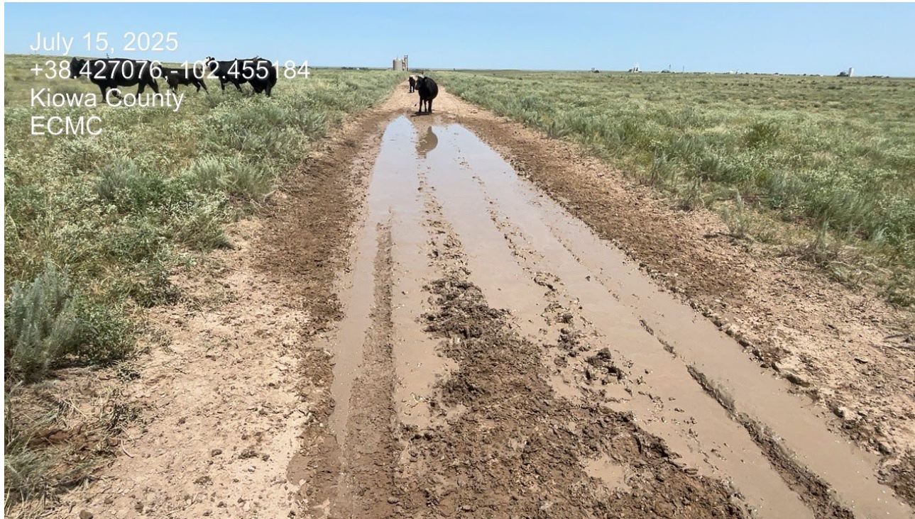
Photo 2. Facing north along the access road. Stormwater needs to be diverted off the road. Areas accumulating stormwater need to be built up with BMP's such as roadbase and gravel.
