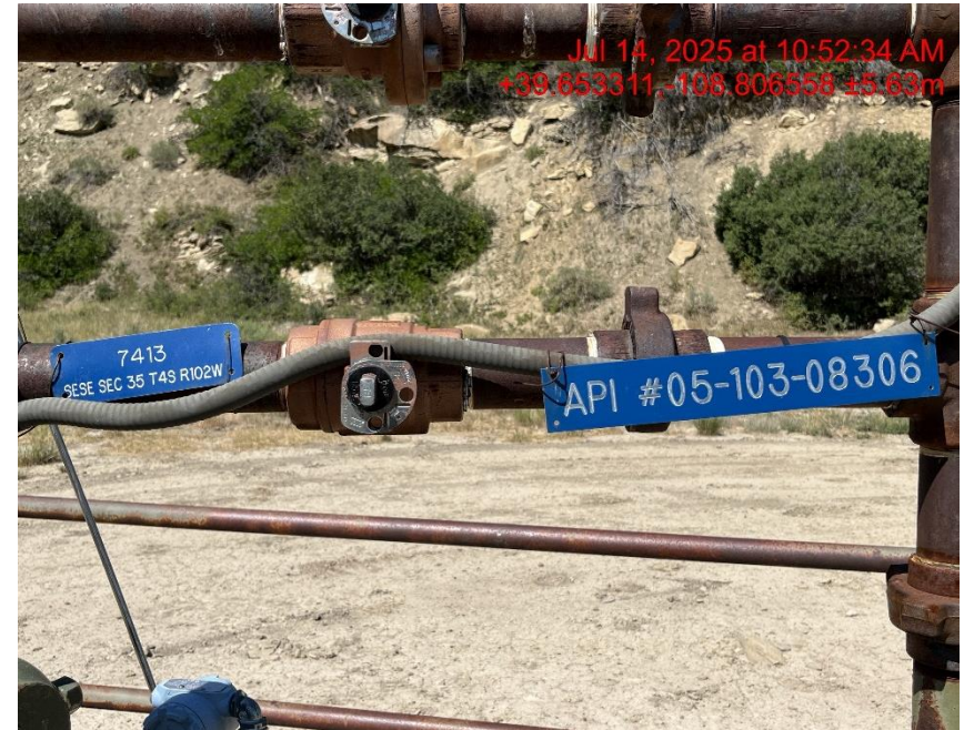
Photo # 9761 Wellhead sign lacks required information/not in compliance with CECMC rules
