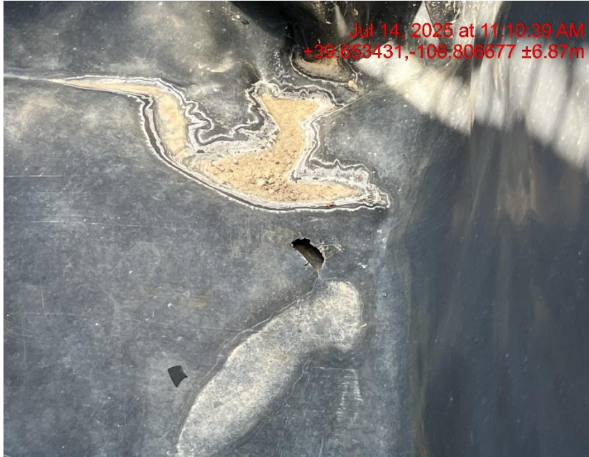
Photo # 9784 Multiple holes/tears in secondary containment liner/liner needs maintenance/liner lacks integrity
