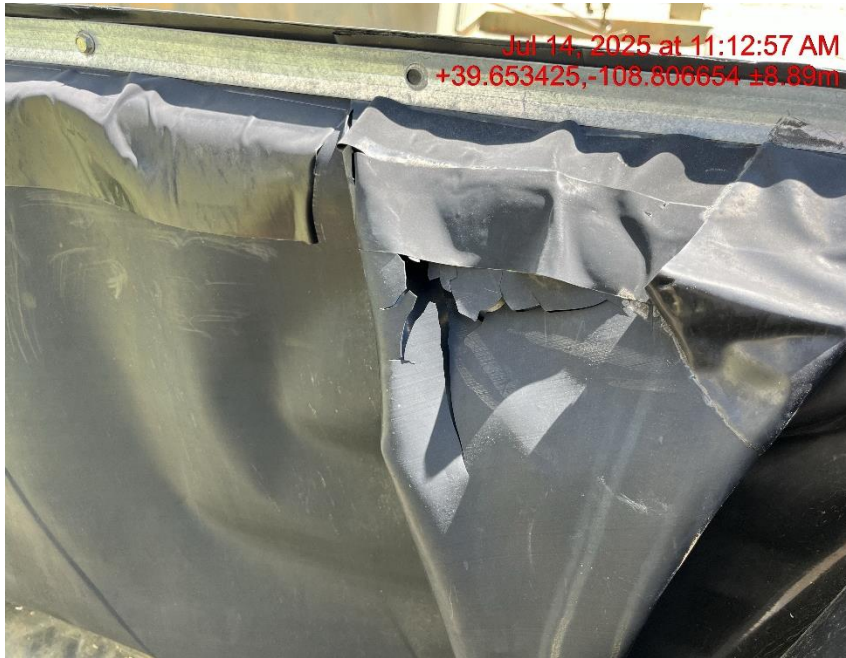
Photo # 9788 Multiple holes/tears in secondary containment liner/liner needs maintenance/liner lacks integrity
