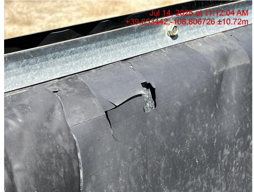
Photo # 9787 Multiple holes/tears in secondary containment liner/liner needs maintenance/liner lacks integrity
