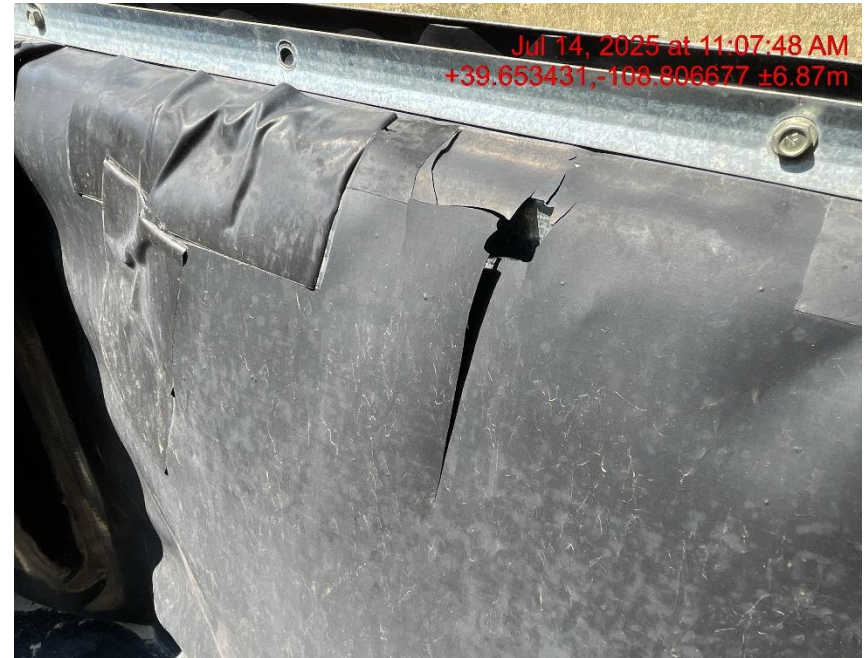
Photo # 9778 Multiple holes/tears in secondary containment liner/liner needs maintenance/liner lacks integrity
