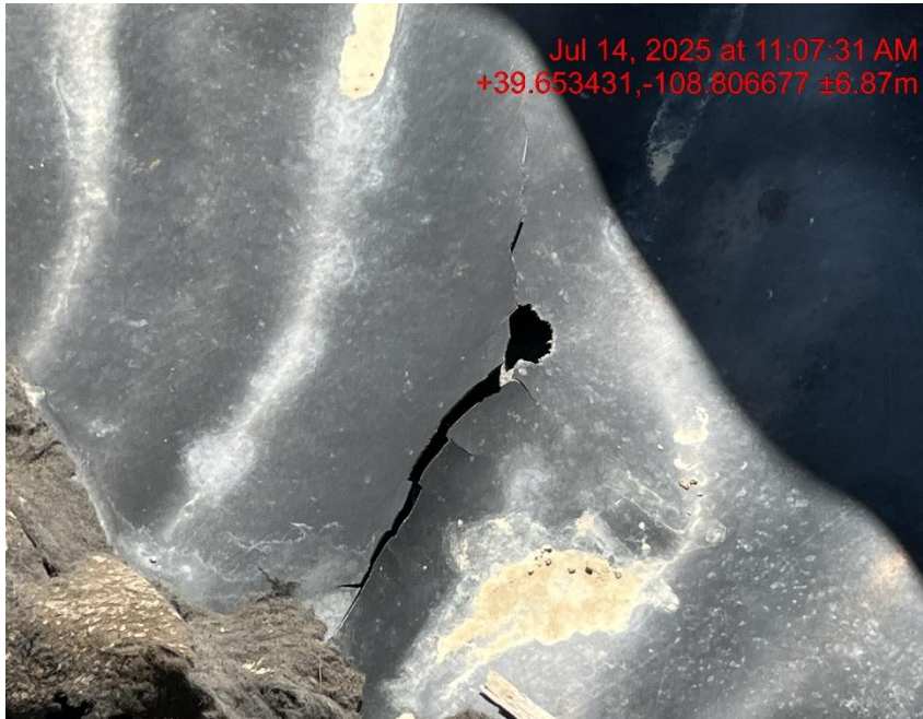
Photo # 9777 Multiple holes/tears in secondary containment liner/liner needs maintenance/liner lacks integrity
