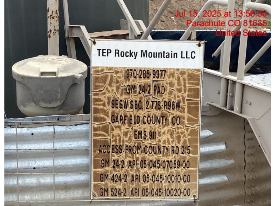
Illegible Battery Sign – Photo #09737
