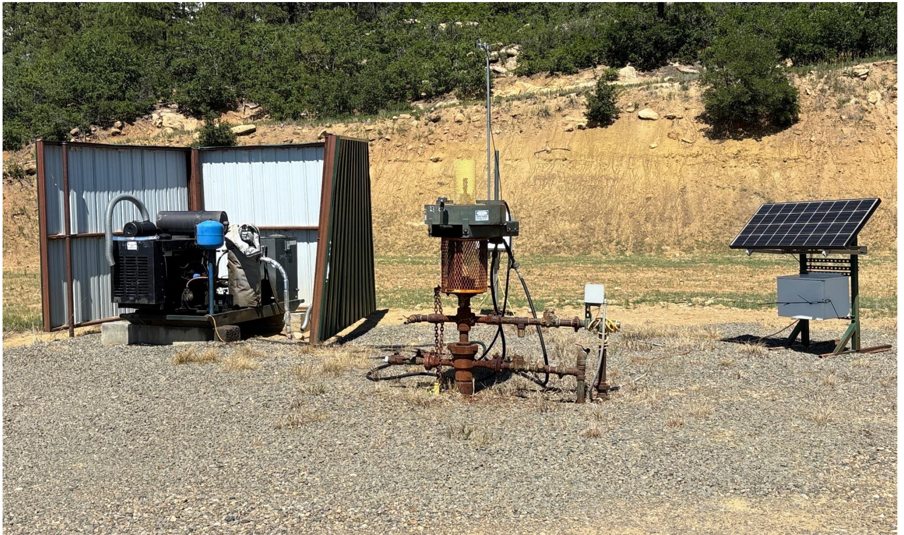
PHOTO 3: WELLHEAD AND EQUIPMENT.
