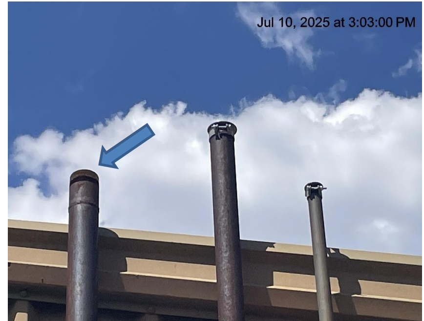
Photo # 1425 PRV vent line does not comply with CECMC pressure safety device rules
