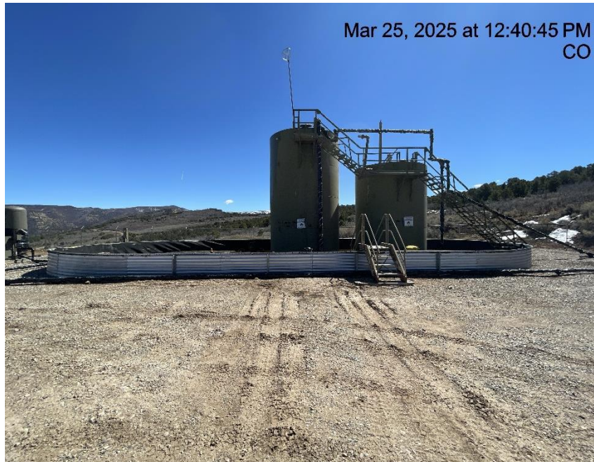
Photo # 7132 From inspection/audit 708906125 conducted on 03/25/2025 Tank battery lacks required signage
