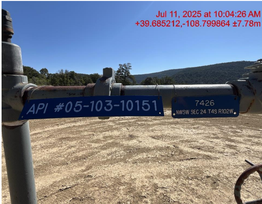
Photo # 9594 Wellhead sign lacks required information/not in compliance with CECMC rules
