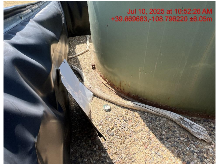
Photo # 9462 Debris on location
