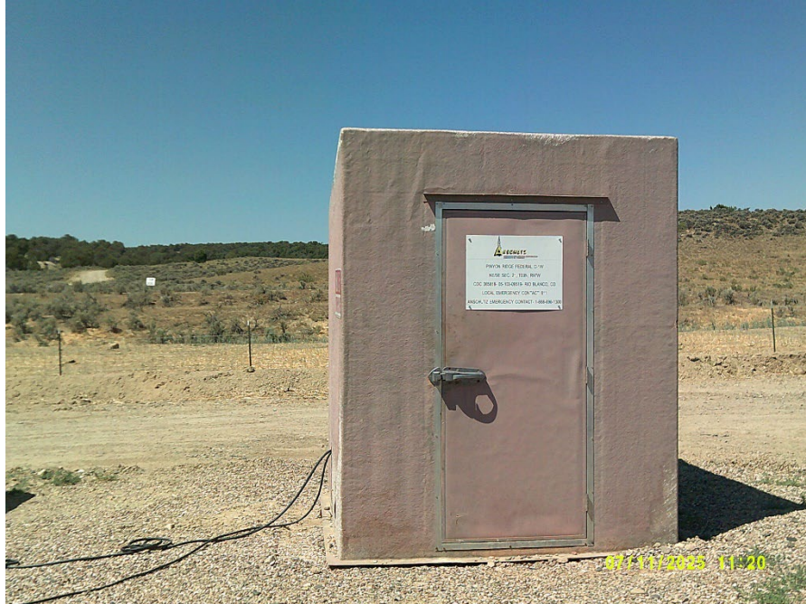
Injection wellhead housing
