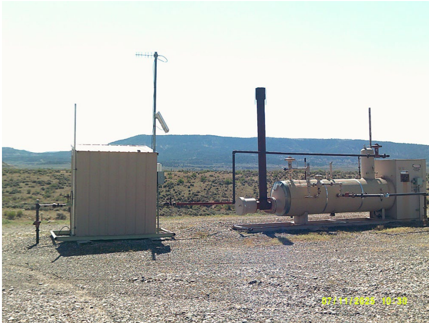
Separator and meter housing
