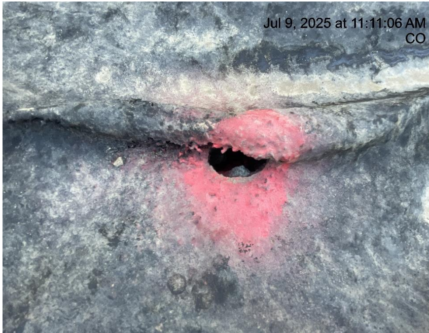
Photo # 102 Hole in liner/liner needs maintenance
