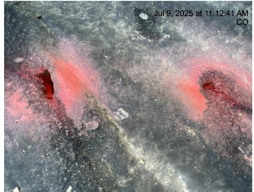
Photo # 107 Holes in liner/liner needs maintenance
