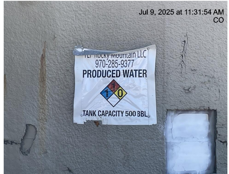
Photo # 111 Tank label starting to peel
