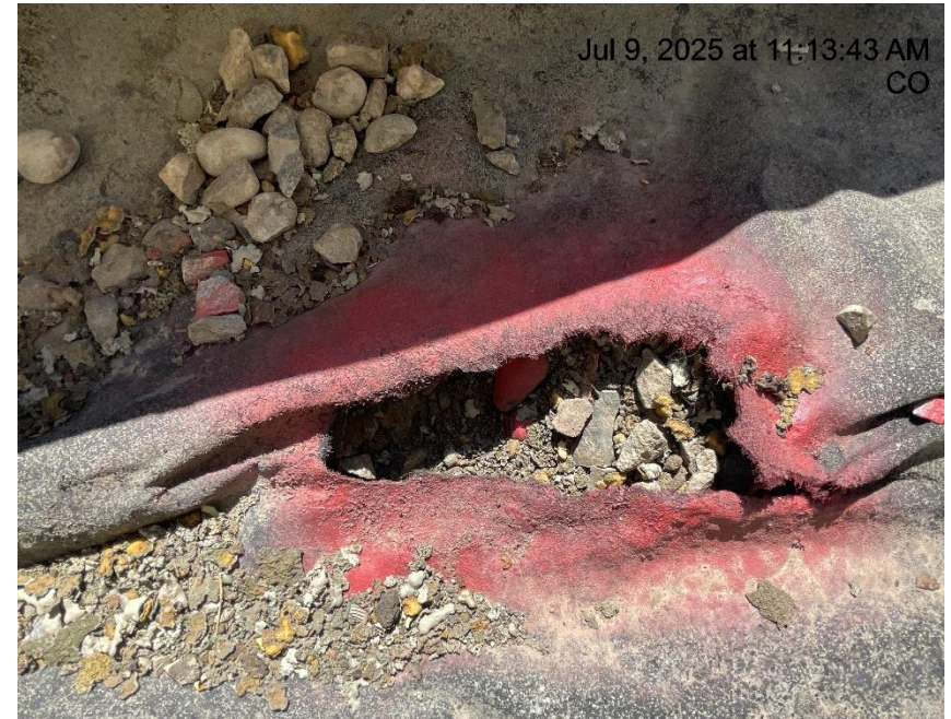
Photo # 109 Hole in liner/liner needs maintenance
