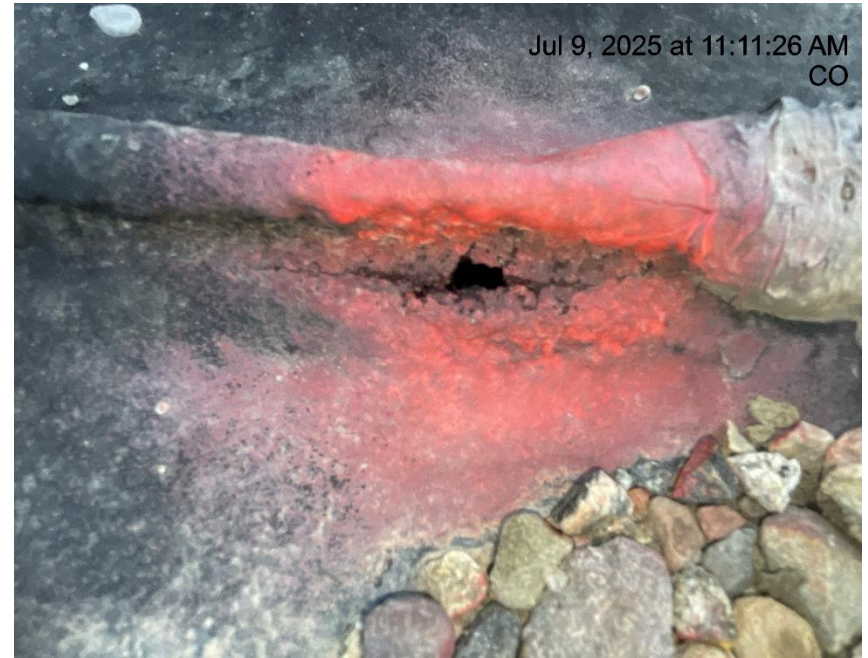
Photo # 103 Hole in liner/liner needs maintenance
