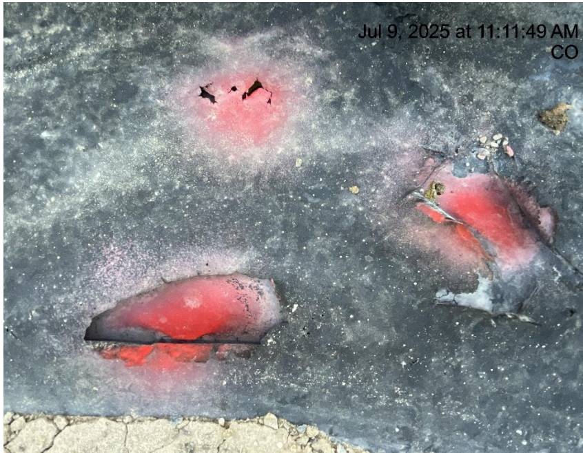
Photo # 104 Holes in liner/liner needs maintenance
