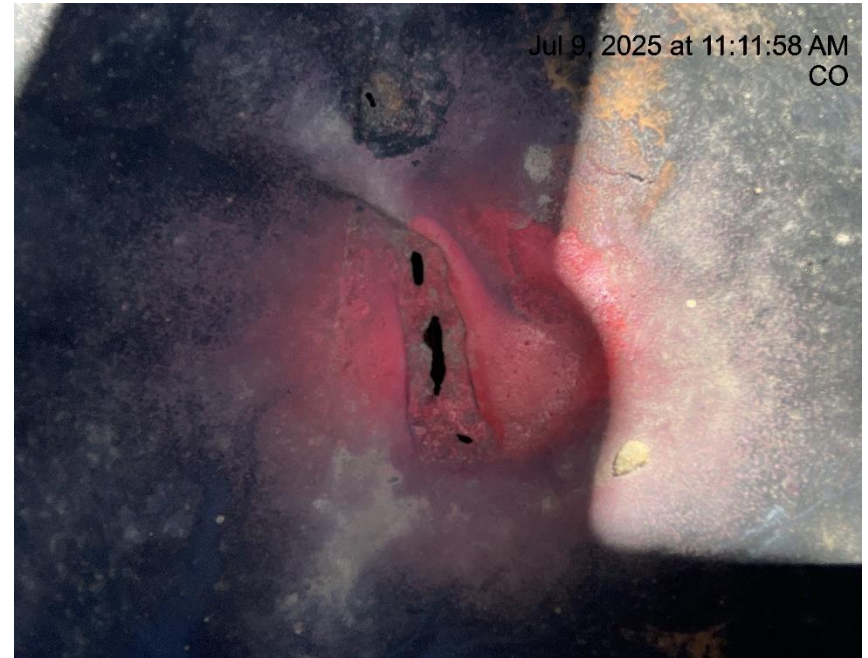
Photo # 105 Hole in liner/liner needs maintenance
