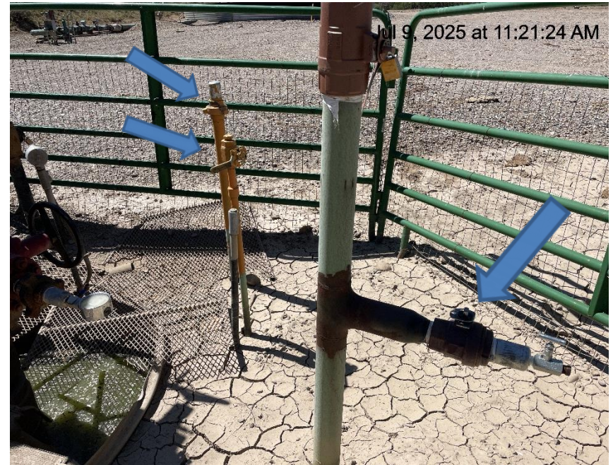
Photo # 101 Unused flowlines lack lockout tagout (OOSLAT)
