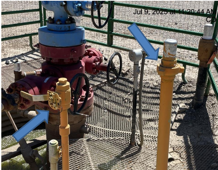
Photo # 100 Unused flowlines lack lockout tagout (OOSLAT)
