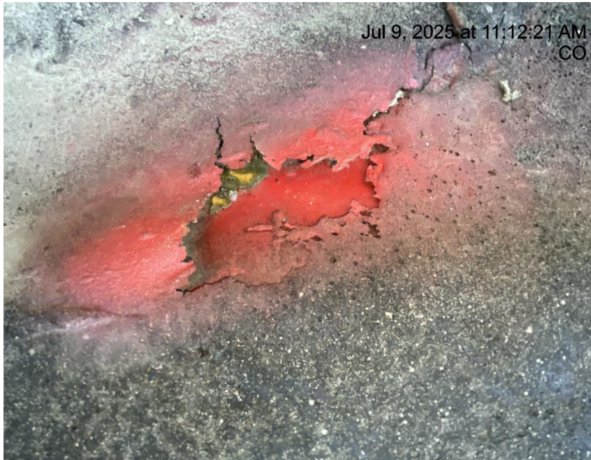
Photo # 106 Hole in liner/liner needs maintenance
