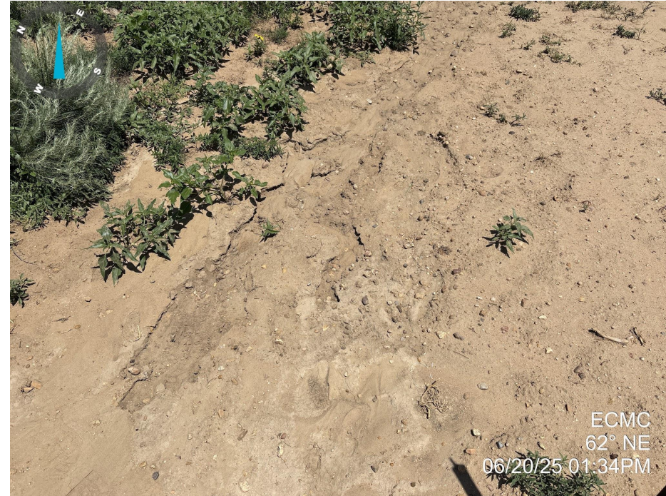
Photo 8. Photo taken of the access road. Photo illustrates stormwater erosion.
