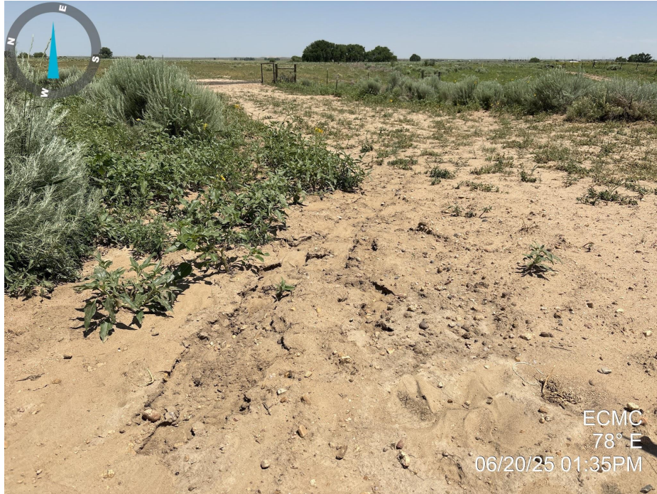
Photo 7. Photo taken of the access road to the well location, facing east. Photo illustrates stormwater erosion along the access road.
