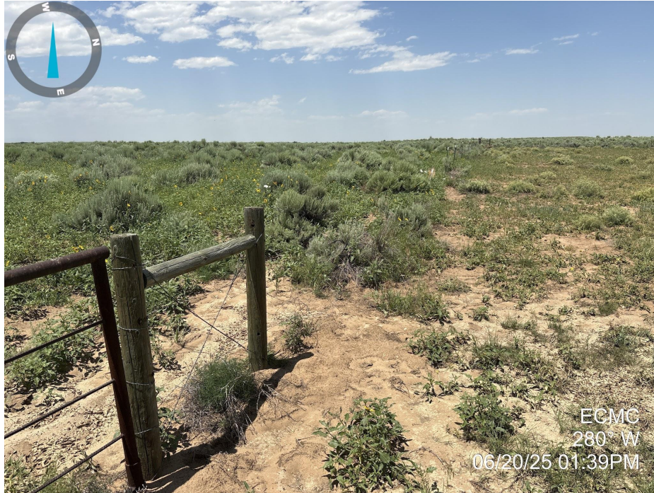
Photo 9. Photo taken from the entrance to the well location, facing west. Photo illustrates fencing remains in place, but is in disrepair.
