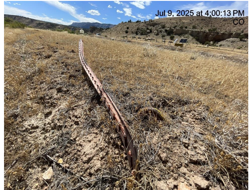
Photo # 367 Same improperly marked deadman
