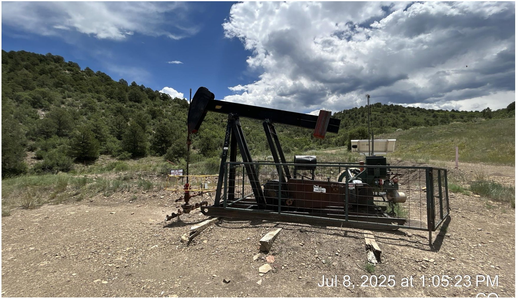
PHOTO 3: WELLHEAD AND EQUIPMENT
