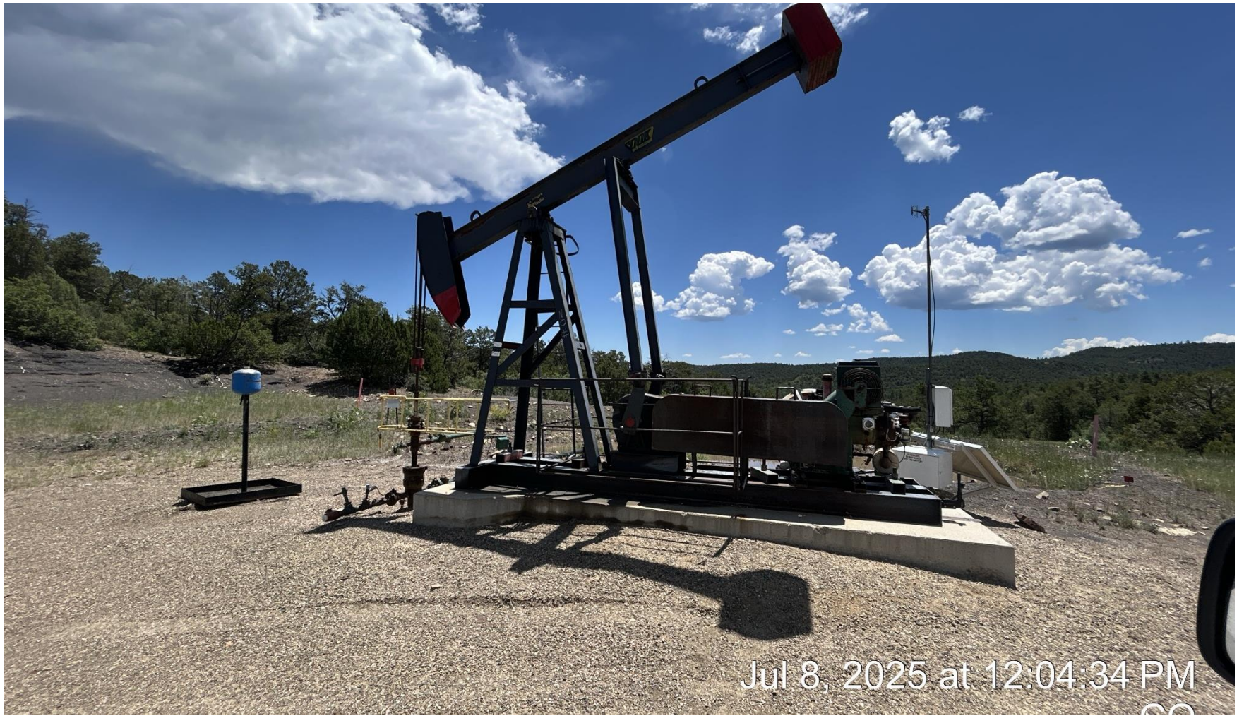
PHOTO 3: WELLHEAD AND EQUIPMENT
