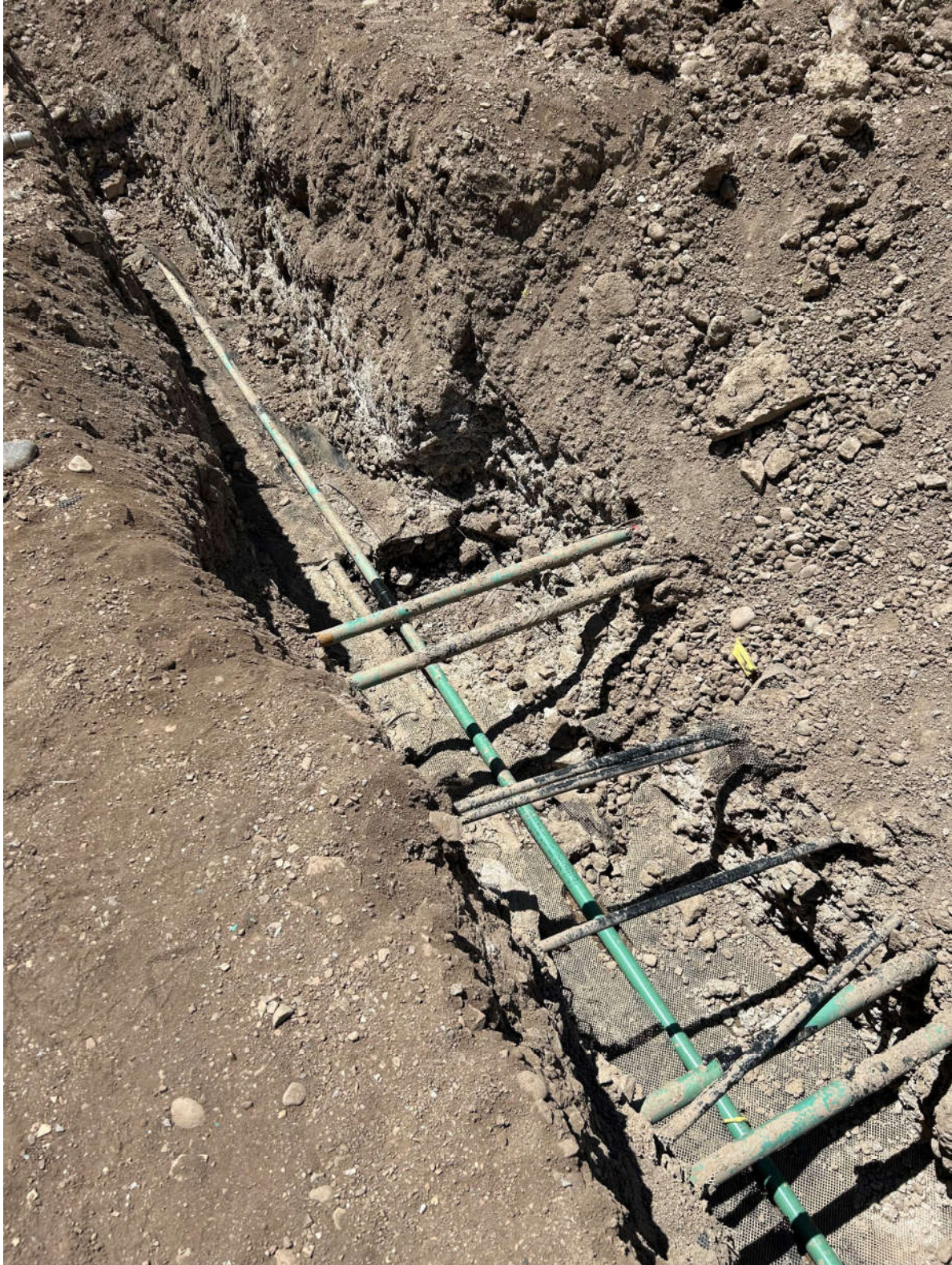
H17 (4A-16) flowline release point within excavation
