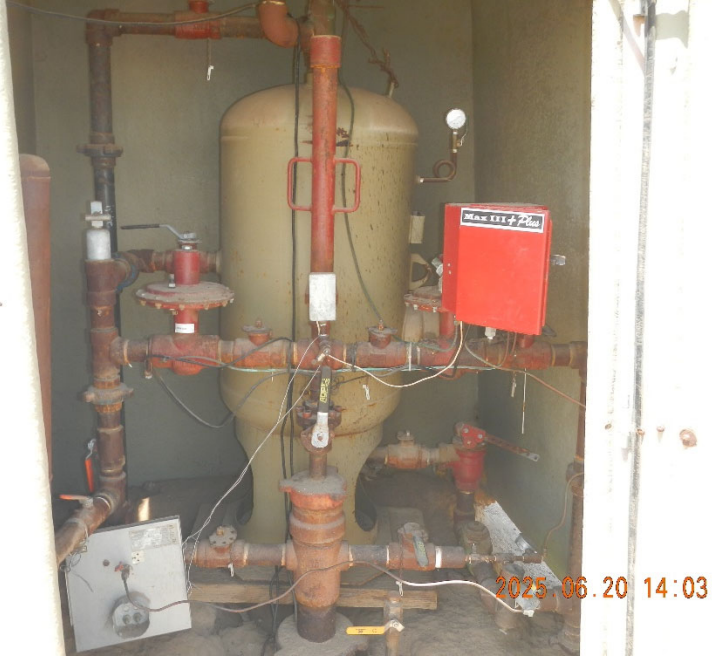
3. View of equipment inside well house.
