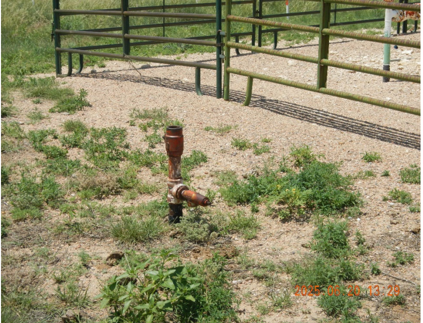
7. Flow line riser with valve missing plug outside fencing at remote gathering location.
