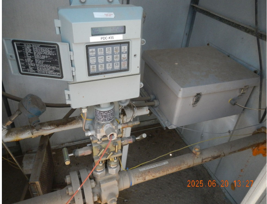
6. Gas meter inside meter shed
