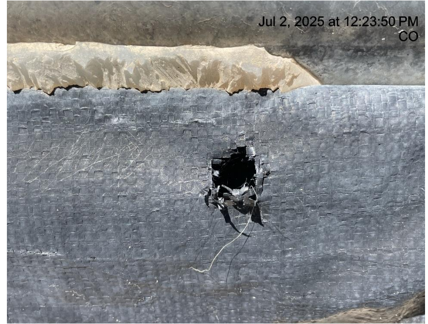
Photo # 9384 Hole in liner/liner needs maintenance
