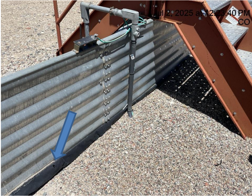
Photo # 9383 Hole in liner/liner needs maintenance
