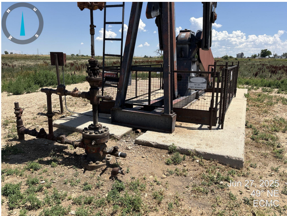
Photo 3. Picture taken at the wellhead. The well is shut in at the time of inspection.
