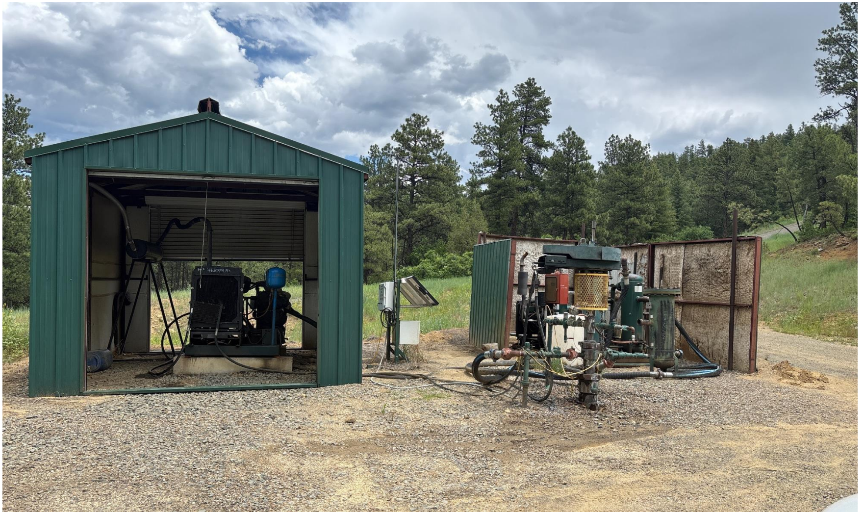
PHOTO 3: WELLHEAD AND EQUIPMENT.
