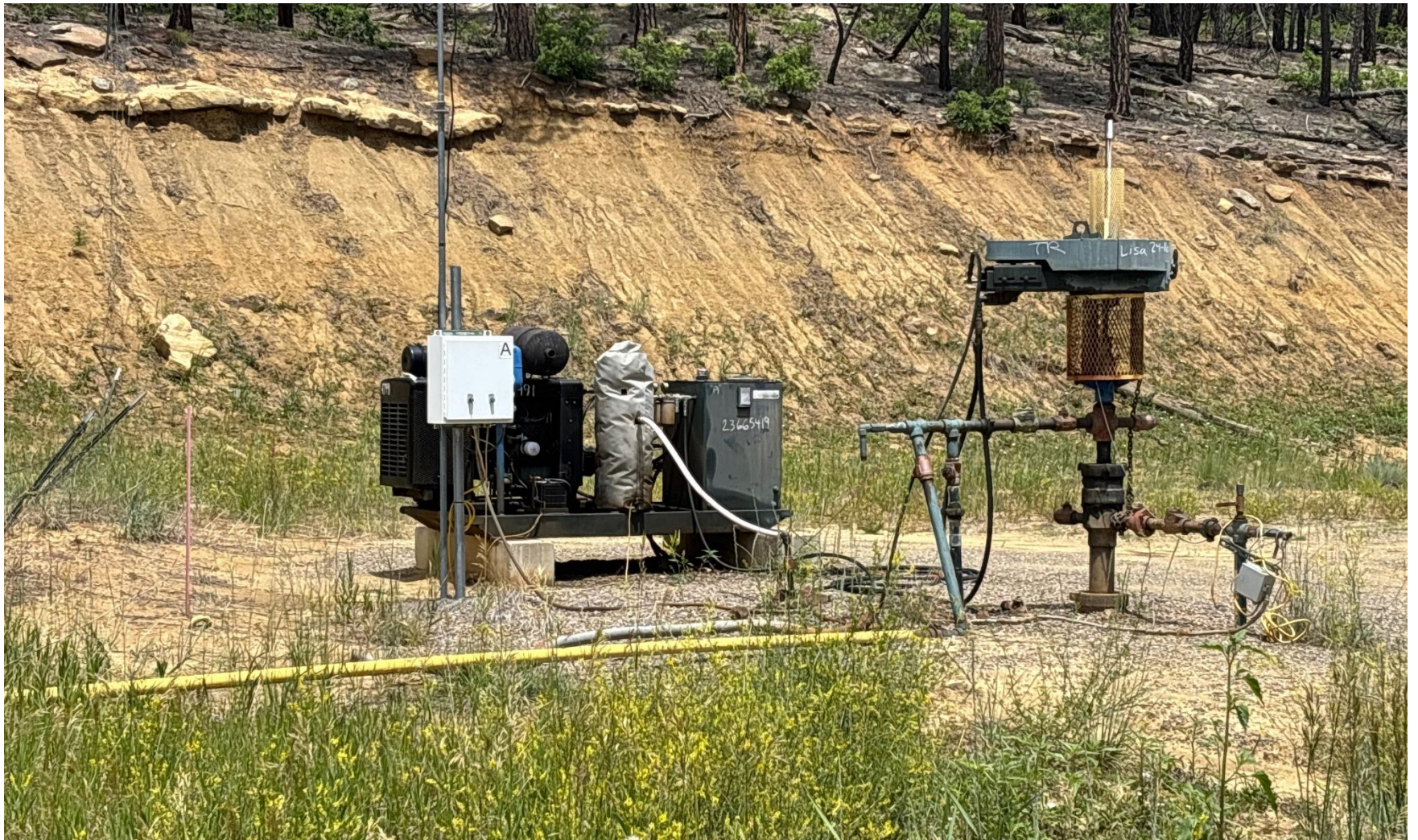
PHOTO 4: TR WELLHEAD AND EQUIPMENT.
