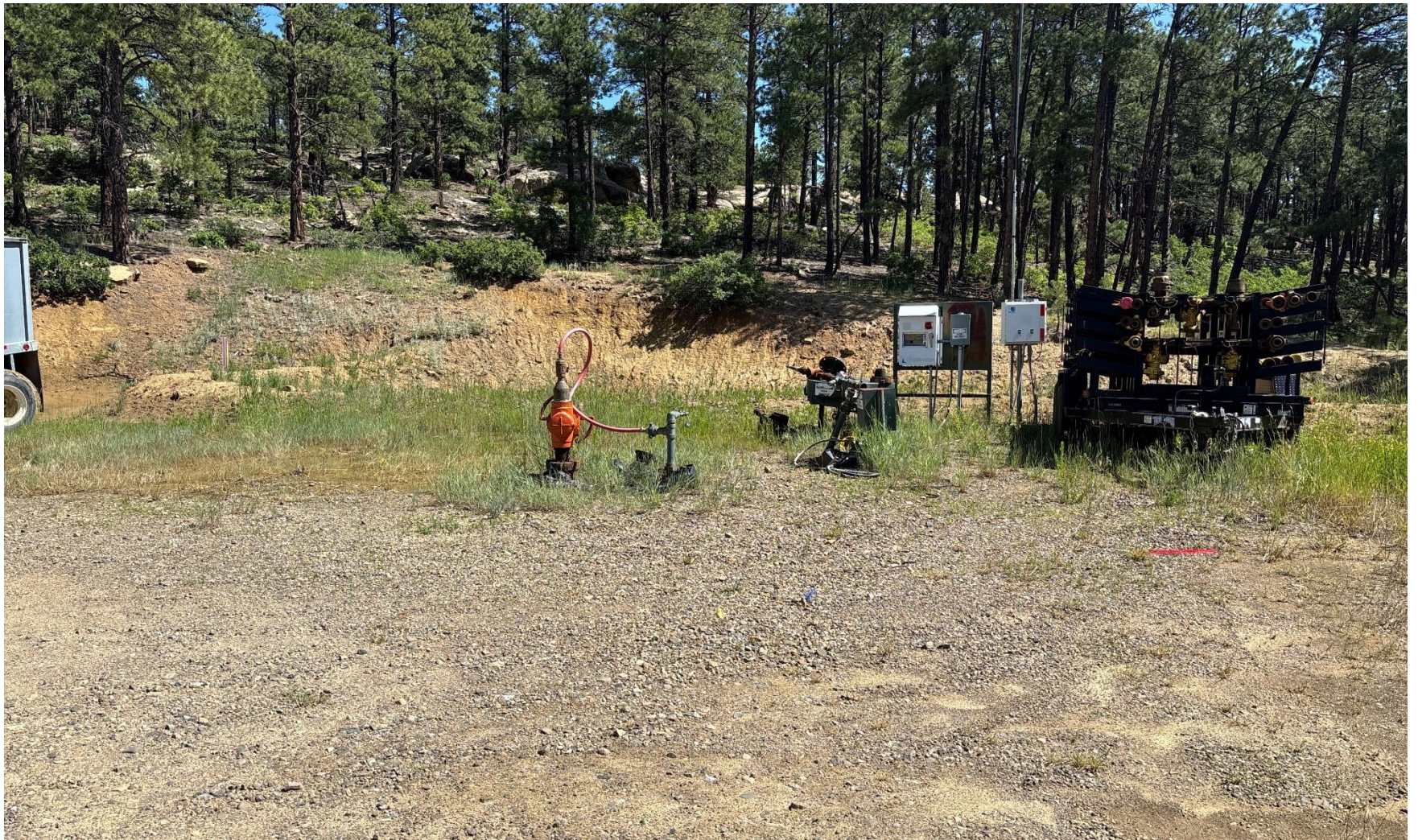
PHOTO 3: WELLHEAD AND EQUIPMENT.
