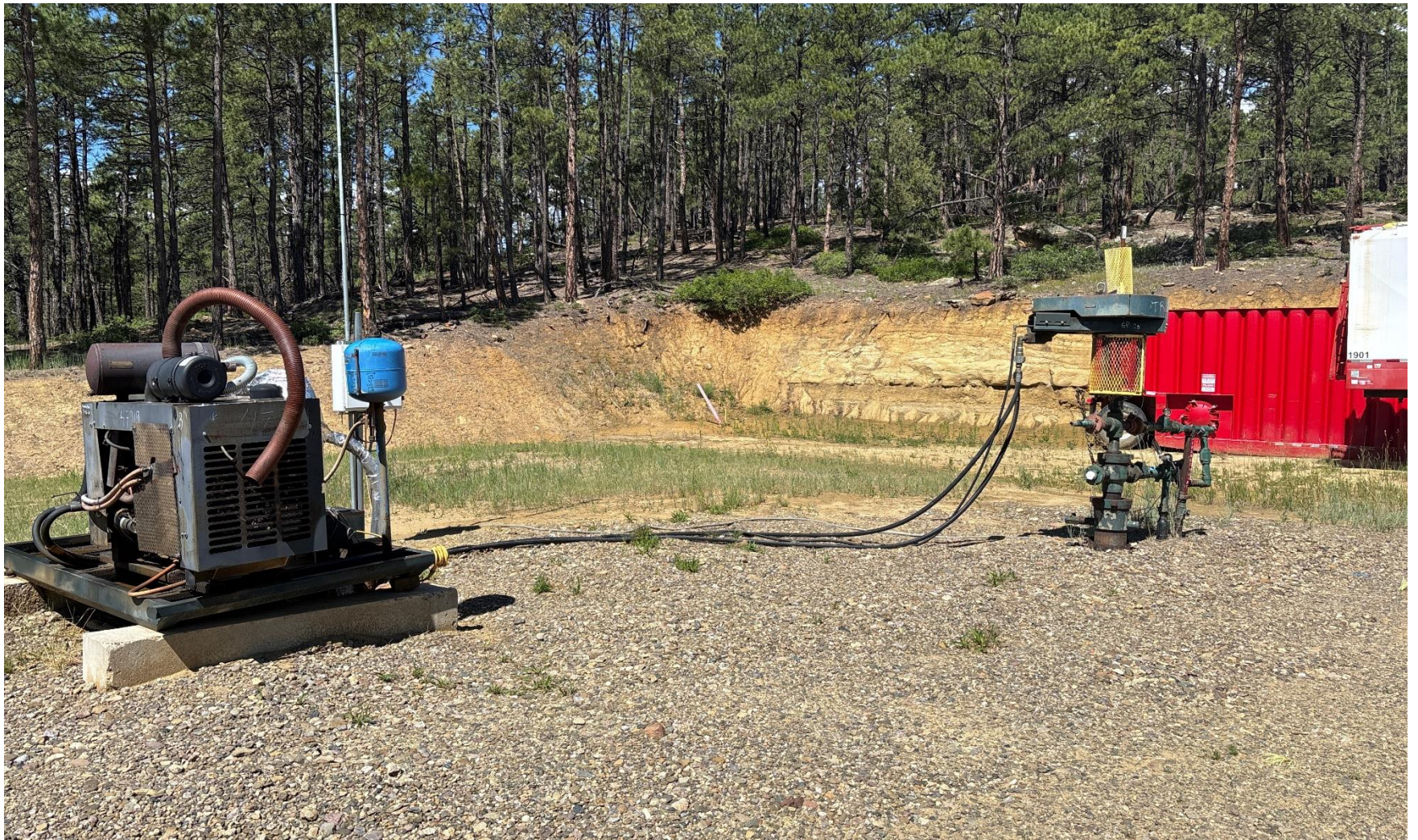
PHOTO 4: TR WELLHEAD AND EQUIPMENT.
