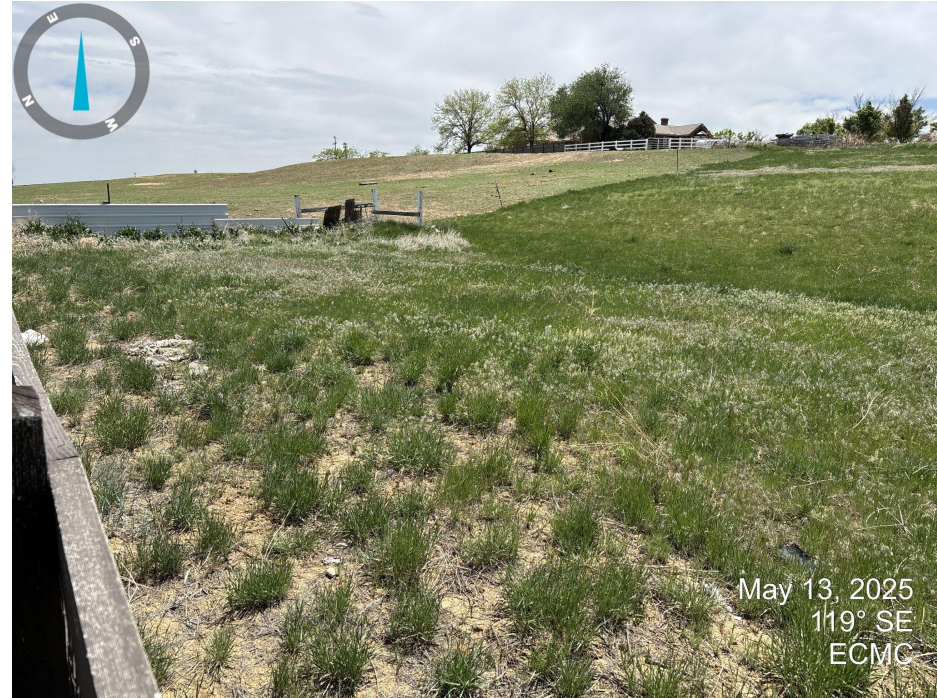
Photo 2. Looking at the southeast part of the well location from center. Vegetation coverage appears to be 80% of the reference vegetation.
